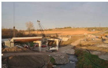
A video of the Keg Creek bridge installation project features time-lapse imagery of the construction.
