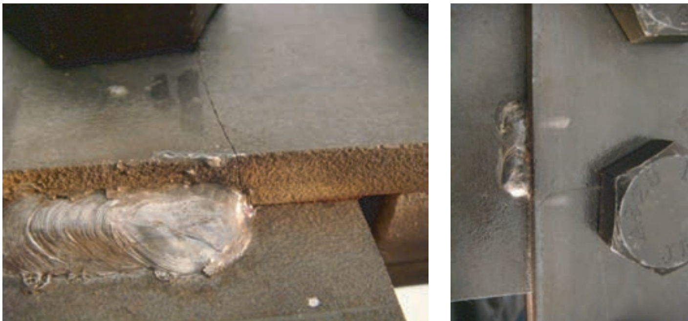
Figure 41. Typical tack weld cracks.
