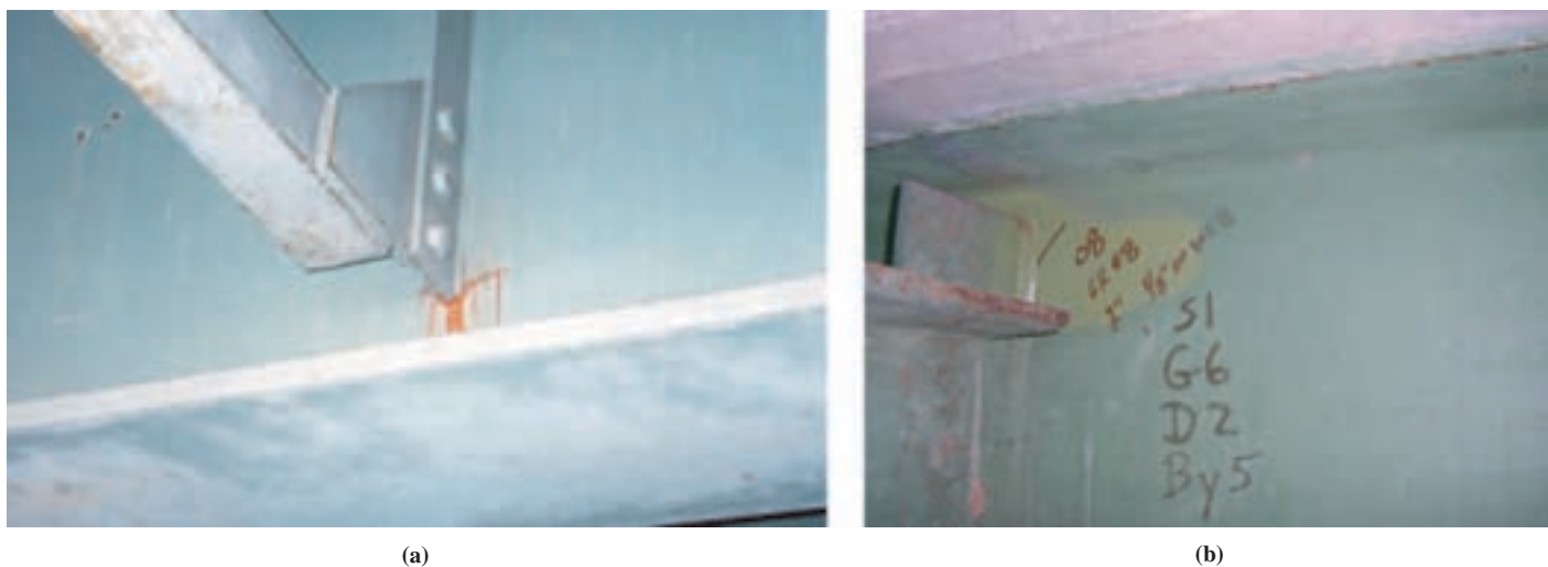
Figure 4. Distortion-induced fatigue cracking at (a) lower end of vertical connection plate and (b) upper end of connection plate.
