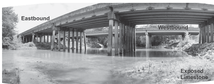
Figure 3.25. I-10 Bridge over Chipola River—view looking upstream. The bridge is straight despite the curved appearance caused by several photographs being merged into a single image.
