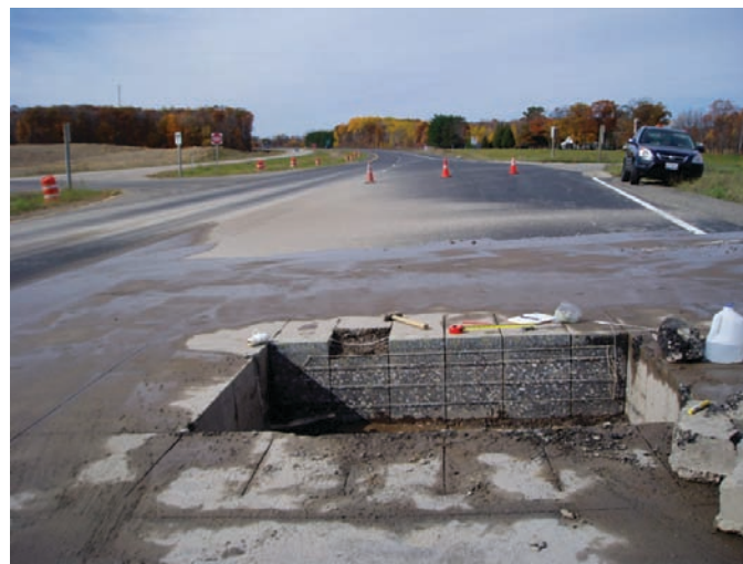
Trench excavated from Wisconsin test section 55-0116. This test section had the greater measured rut depth and included the asphalt-treated base layer.
