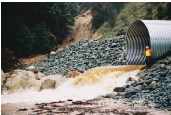
Figure 4-1. Culverts of less than 20 feet in span are routinely inspected in many states ( http://www2.dot.ca.gov/hq/oppd/dib/dib83-01-4.htm ).
