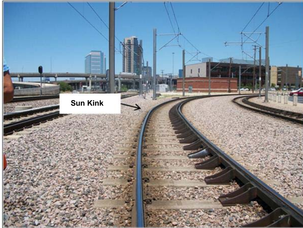
Figure 41. Sun Kink Observed During Track Inspection
