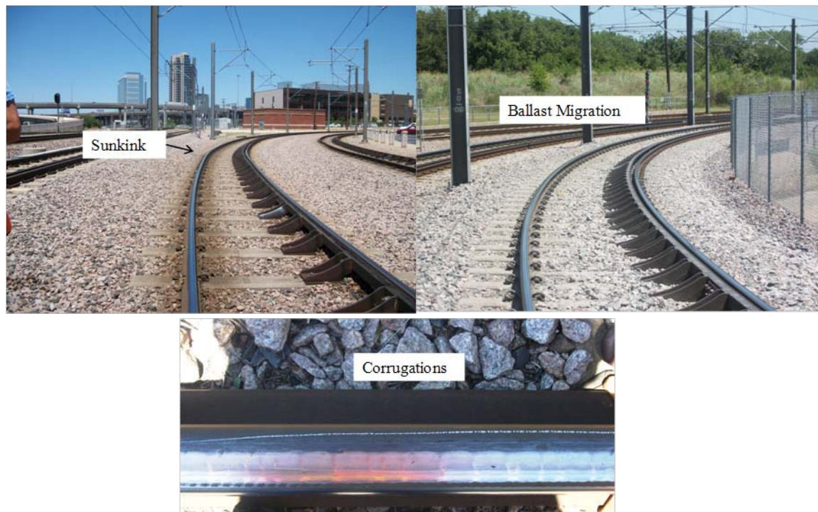
Figure 13. Track Geometry Issues
