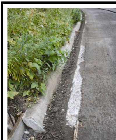
Figure 5.6. On the Historic Columbia River Highway, the removal of generations of asphaltic overlay brought back to the original Warrenite pavement (lighter color), an early 20th century proprietary bitulithic paving material. This has also allowed for the restoration of the concrete gutter system. Photo courtesy Robert Hadlow, Oregon DOT.
