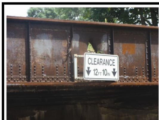
Figure 5.14. There are advantages for posting vertical clearance signs in advance of the obstruction. They can prevent overhead bridges that contribute to historic districts from being physically damaged by oversized vehicles. It does little good to place warning signs after the overhead obstruction has been hit. Photograph M. McCahon
