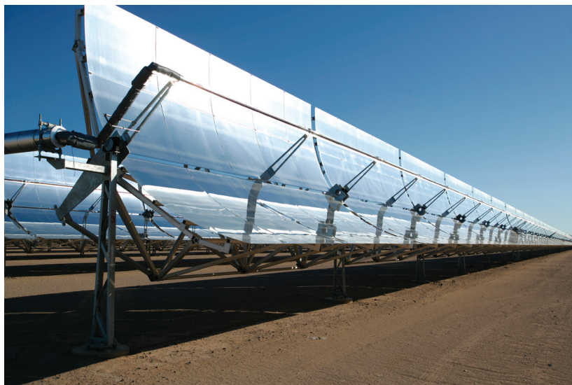
FIGURE 5.10 A parabolic trough concentrator solar thermal plant in Nevada. SOURCE: Courtesy of Acciona Solar Power.
