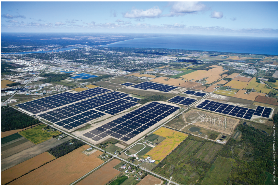
FIGURE 5.6 Eighty-megawatt thin-film cadmium telluride (CdTe)-based solar plant in Canada. SOURCE: Courtesy of First Solar.
