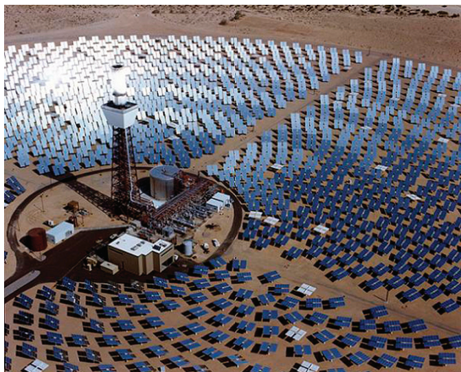
FIGURE 5.2.1 In this photograph of a concentrating solar power (CSP) technology, stretched membrane heliostats with silvered polymer reflectors will be used as demonstration units at the Solar Two central receiver. The Solar Two project will refurbish this 10-megawatt central receiver power tower, known as Solar One. SOURCE: Image available at https://www.eere.multimedia.energy.gov/solar/ .
