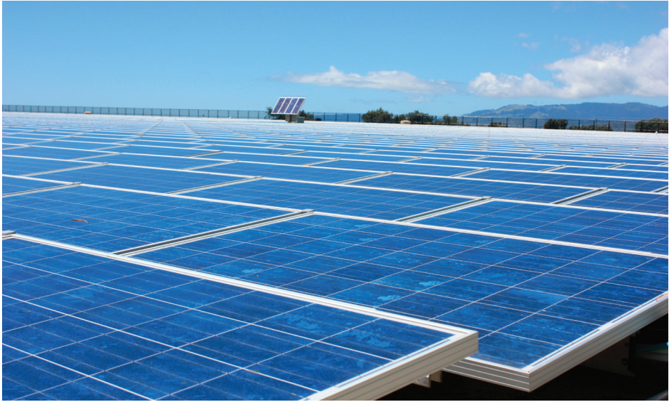
FIGURE 5.5 Silicon solar cells deployed for utility power production. SOURCE: Courtesy of Suntech Power Holdings, Inc.
