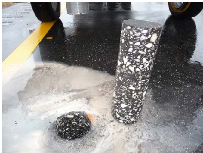
Figure 1.34. Core 3 from Station 1+35 in Section 5.
