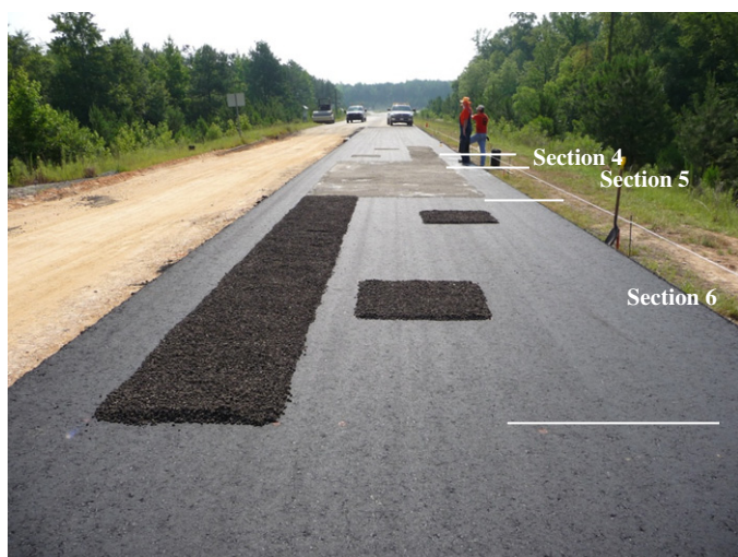
Figure 1.27. Approximately 1-in.-thick, uncompacted RAP materials placed in Section 6 at depth of 2 in.
