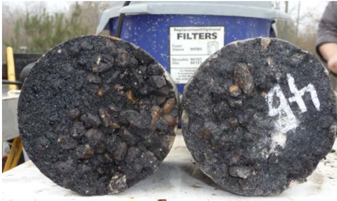
Figure 1.35. Core 4 from Station 2+10 in Section 8.
