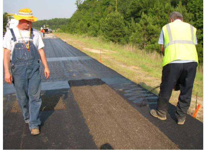
Figure 1.24. Uncompacted RAP material approximately 1 in. thick placed in Section 8 at depth of 5 in.
