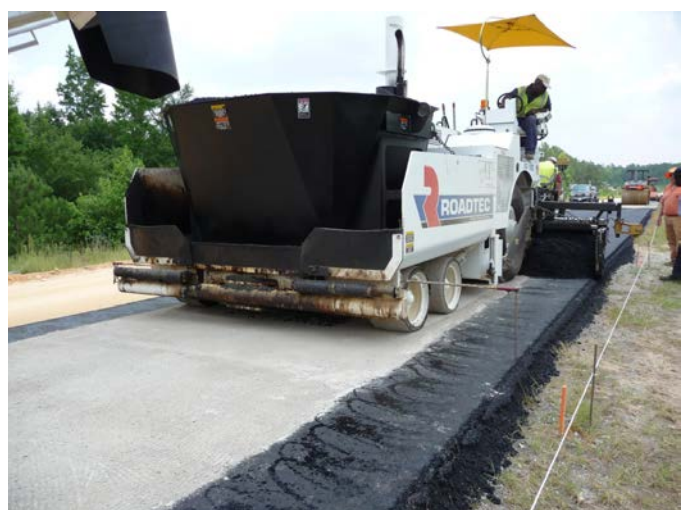
Figure 1.29. Paver placing 2-in. surface lift over baghouse fines in delaminated area in Section 5.
