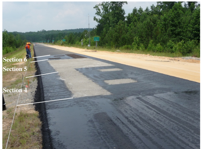
Figure 1.28. Baghouse fines used as bond breaker in Sections 4 and 5 at depth of 2 in.
