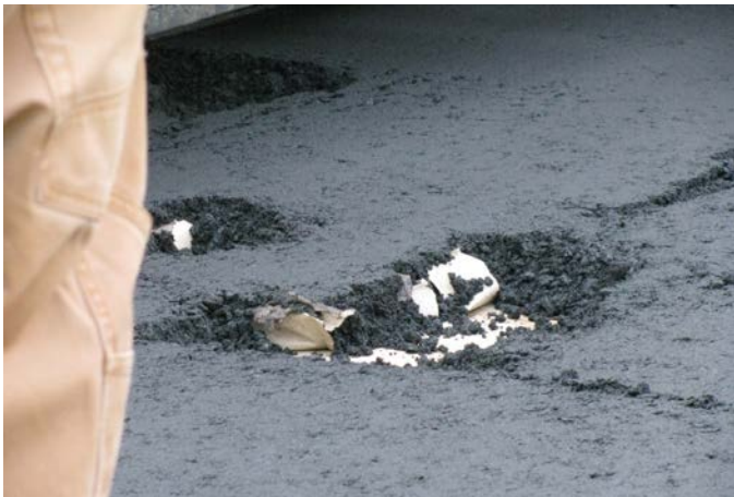
Figure 1.26. Brown paper torn by paver at one location in Section 9.
