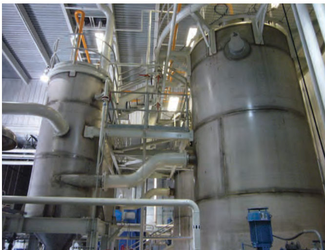
Figure 2. Biological reactor units (at right) in the CAK AFBR system.
