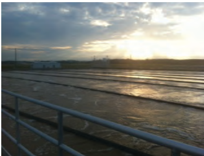
Figure 3. The airport's activated sludge treatment system aeration basins (Photo courtesy of KCAB).
