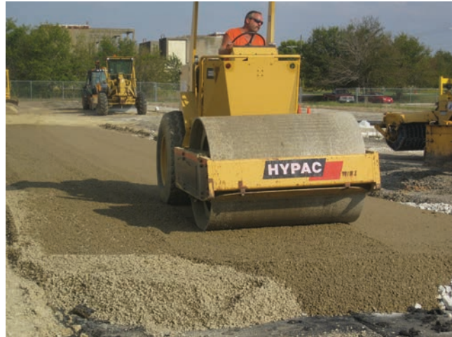
FIGURE 79 Compaction of a crushed limestone base course using a smooth drum vibratory roller.
