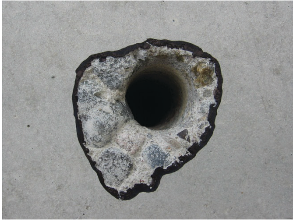
Figure 12: Chipped area around top of hole.
