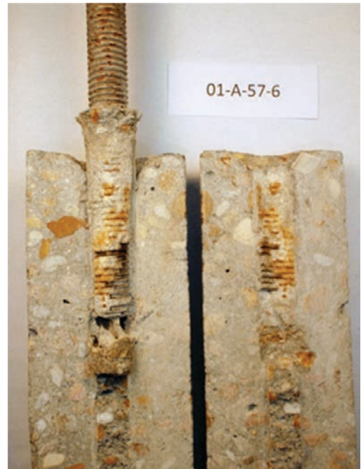
Figure 50. Typical shearing failure at threads.
