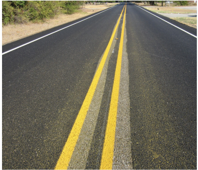
Figure 33. Water blasted thermoplastic on new asphalt surface (away from sun).
