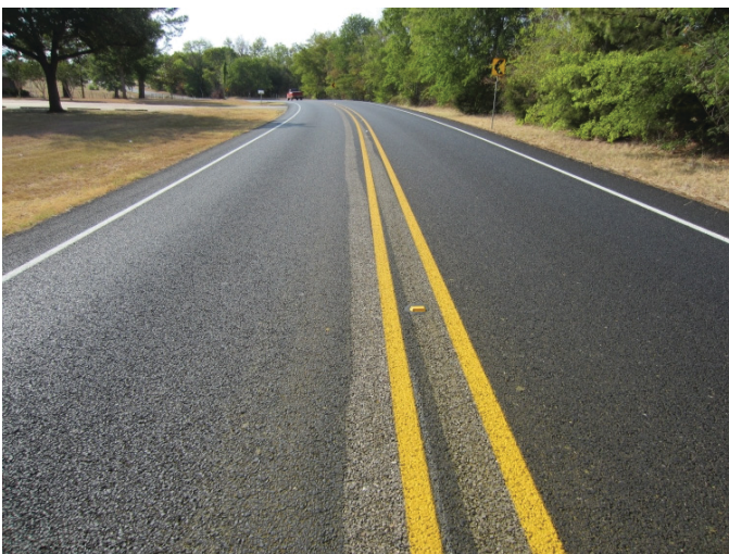
Figure 32. Water blasted thermoplastic on new asphalt surface (toward sun).
