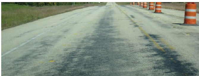
b) Insufficient marking removal and poor temporary markings.
