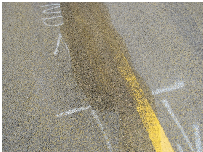
Figure 36. Water blasted thermoplastic on asphalt surface (close view).
