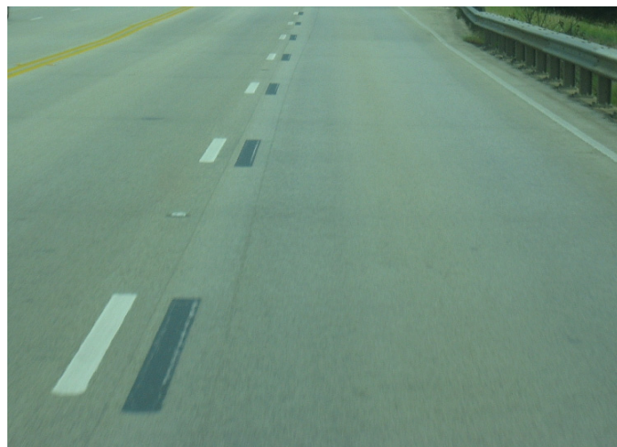
Figure 55. Black marking material covering old marking.
