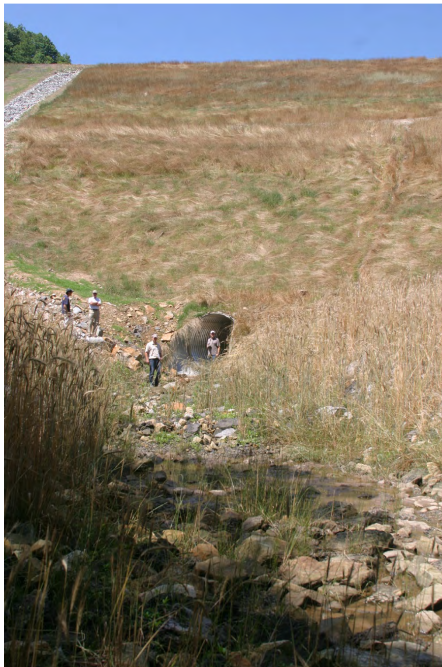
Figure 4.1. The outlet of a culvert crossing beneath a section of the Coalfields Expressway.
