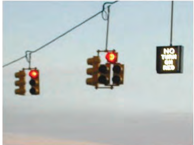
FIGURE 6 Dynamic no-turn-on-red installation in Livingston County, Michigan. Source: Hughes et al. 2006.
