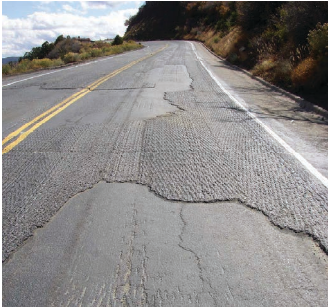
Figure 3. Milled pavement surface with thin scab layer which will likely lead to premature failure of the overlay.
