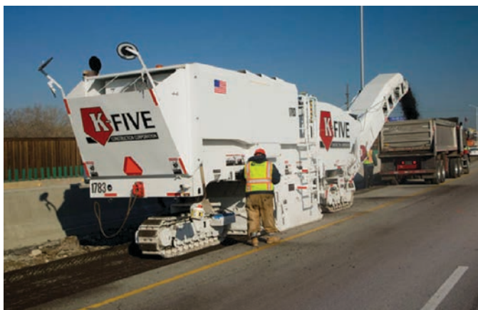
Figure 1. Milling machine removes asphalt pavement layers as part of pavement rehabilitation. (Photo courtesy of Astec Industries.)
