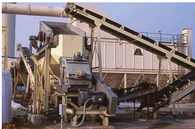
Figure 13. When using in-line RAP crushers, check extracted gradations before and after the crusher to make sure the RAP aggregate gradation is not changing.
