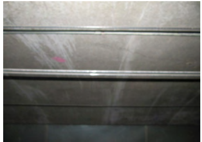
(b) Defective location
