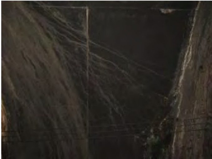
(a) Intact location
