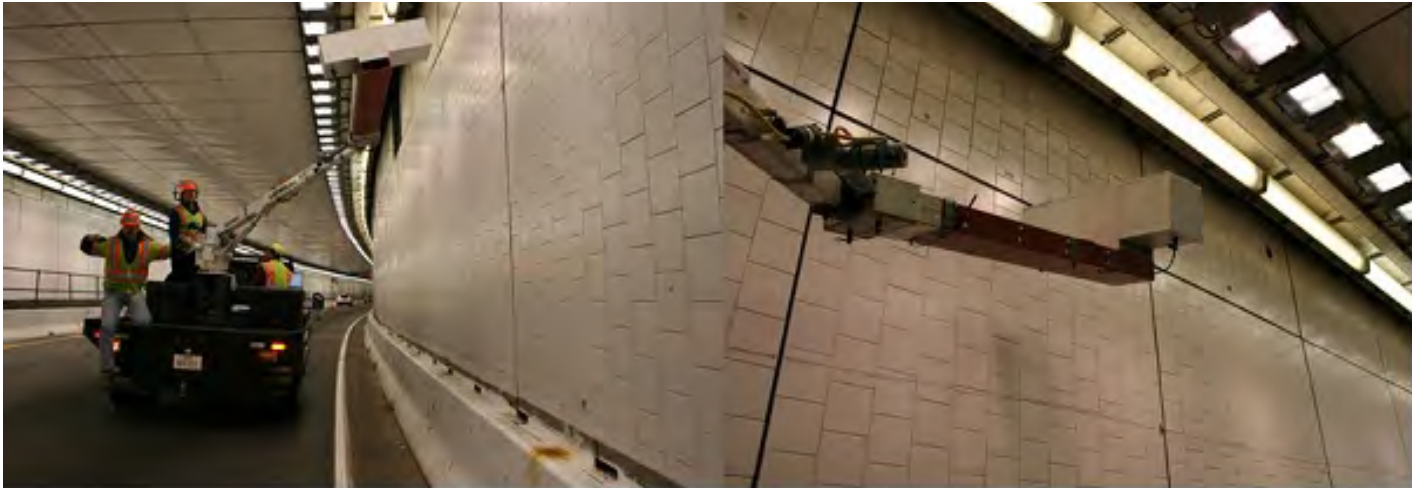
Figure J.14. GPR antenna mounted on a crane. This system, developed and used by Texas A&M Transportation Institute, was used in SHRP 2 U.S. tunnel tests.
