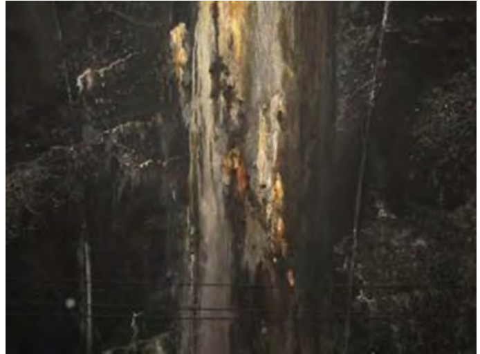
(b) Defective location
