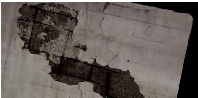
Figure X.3. Liberty Tunnel: Detail of spalling by ventilation shaft.
