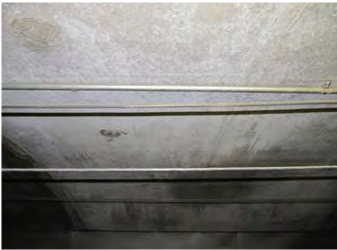
(a) Intact location
