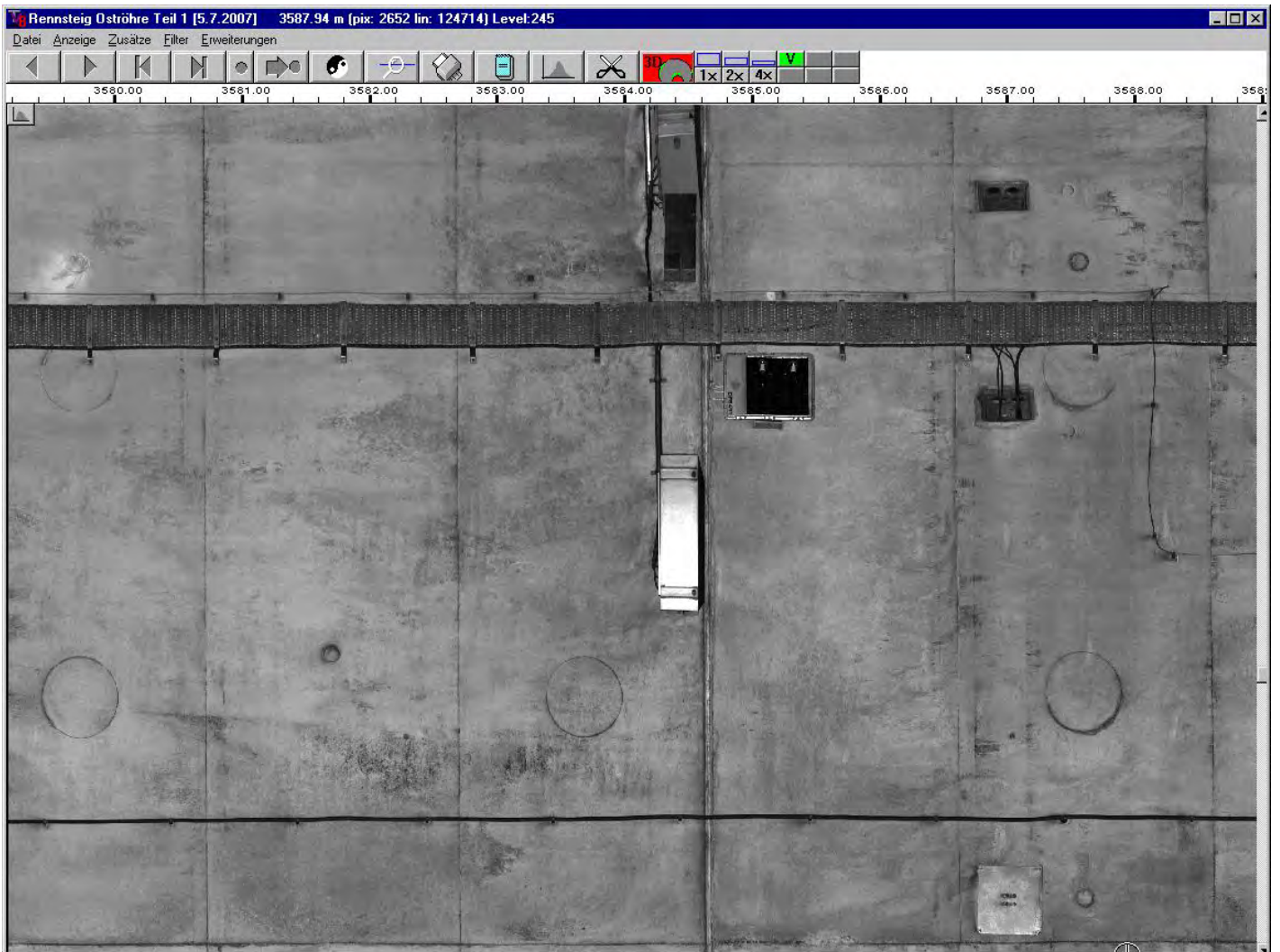
Figure I.3. Visual image of conditions of a shotcrete lining in a motorway tunnel.
