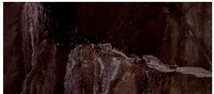
Figure X.21. Clean air supply duct, south-west ventilation building, detail of south lining wall from within duct.
