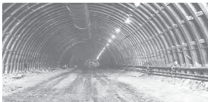
Figure Q.22. Photograph of construction of Eisenhower Memorial Tunnel sometime between 1968 and 1973 (Colorado DOT 2011). Steel beams could be anomaly seen in GPR and ultrasonic echo data.
