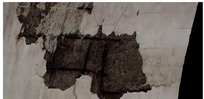
Figure X.4. Foreshortened view of spalling by ventilation shaft.
