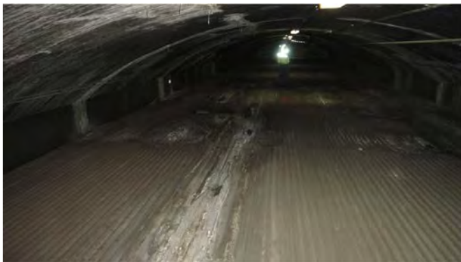
Figure L.25. Visual image of the top of the Hanging Lake Tunnel. Note staining around cracks.
