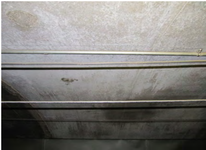
(a) Intact location
