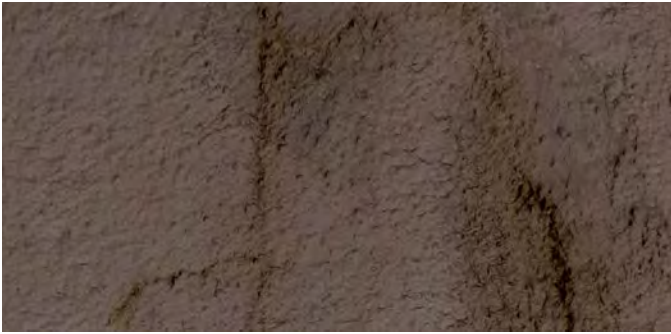
Figure X.12. Detail of shotcrete cracks on left wall by southern portal with digitized cracks toggled off.
