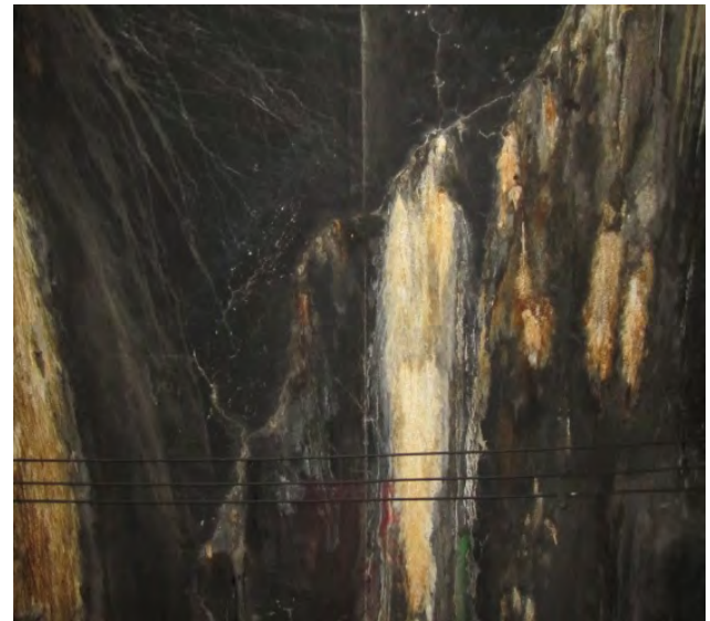
(b) Poor condition
