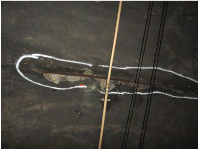
Figure M.47. Typical spalling and corrosion.
