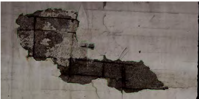
Figure X.7. Closed polyline to determine area of spalling by ventilation shaft.
