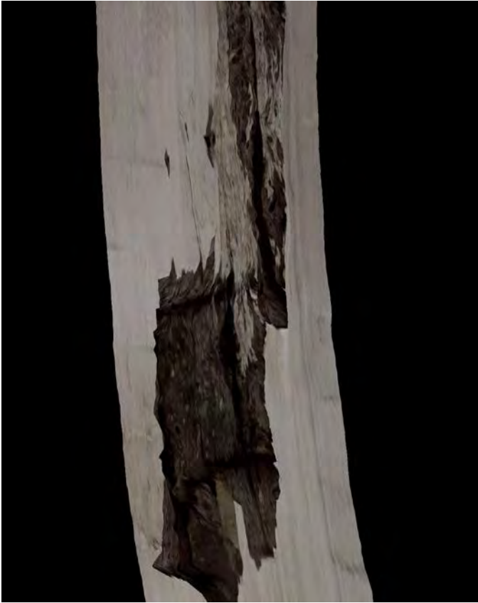
Figure X.6. Backside view of spalling by ventilation shaft to better appreciate depth and extent of spalling.
