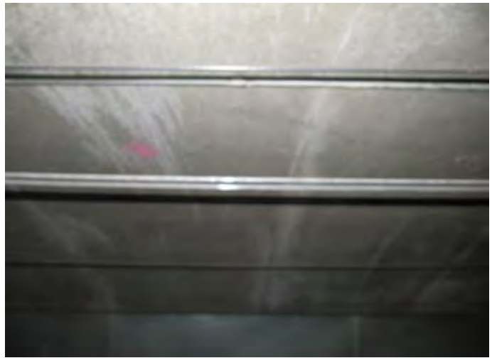
(b) Defective location
