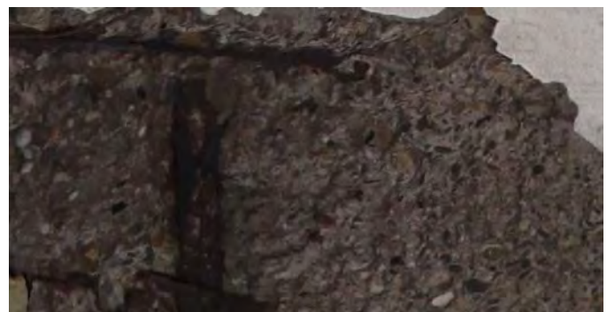
Figure X.5. Detail of exposed aggregate and rebar by ventilation shaft.
