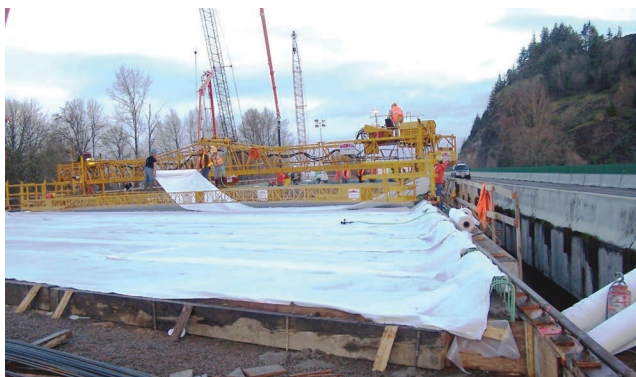
FIGURE 8 Wet curing of a concrete bridge deck under polyethylene sheeting [Photo courtesy of Oregon Department of Transportation].
