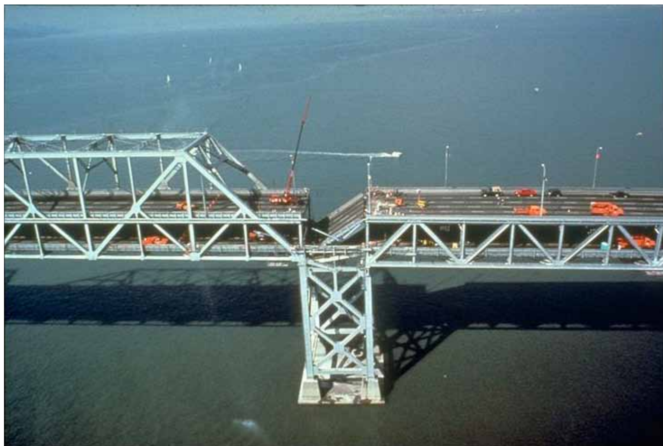
FIGURE 16 San Francisco–Oakland Bay Bridge Span E-9 Collapse, Loma Prieta Earthquake, 1989. (Courtesy: National Information Service for Earthquake Engineering, EERC, University of California, Berkeley.)
