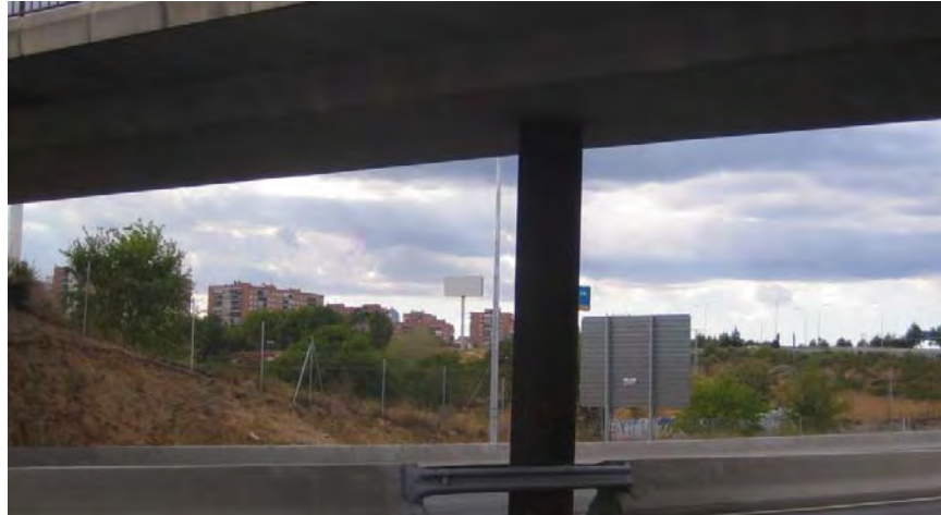
FIGURE 4 Barrier installation is inappropriate.
