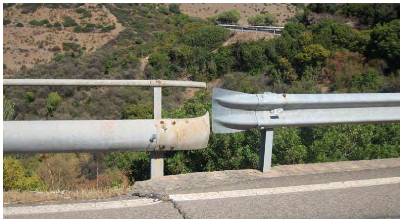
FIGURE 3 Barriers not connected.
