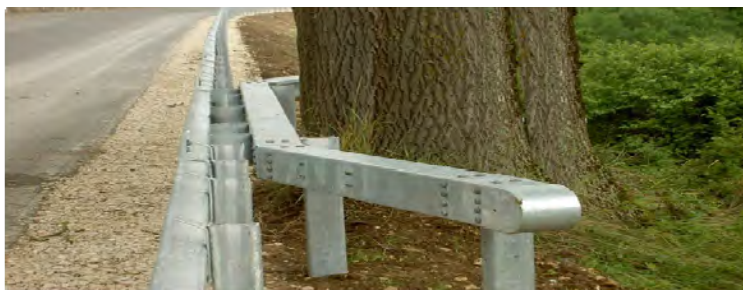
FIGURE 2 Stiffened barrier near a tree.
