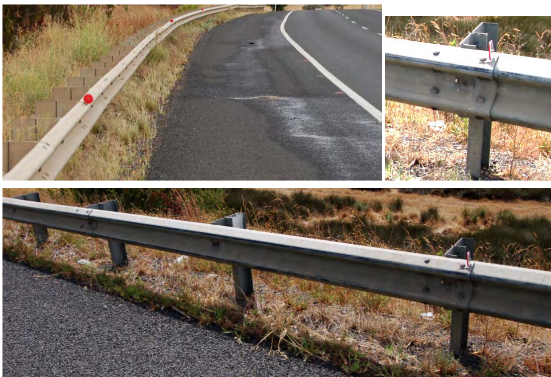
FIGURE 4 W-beam with Charlie post and block-out.
