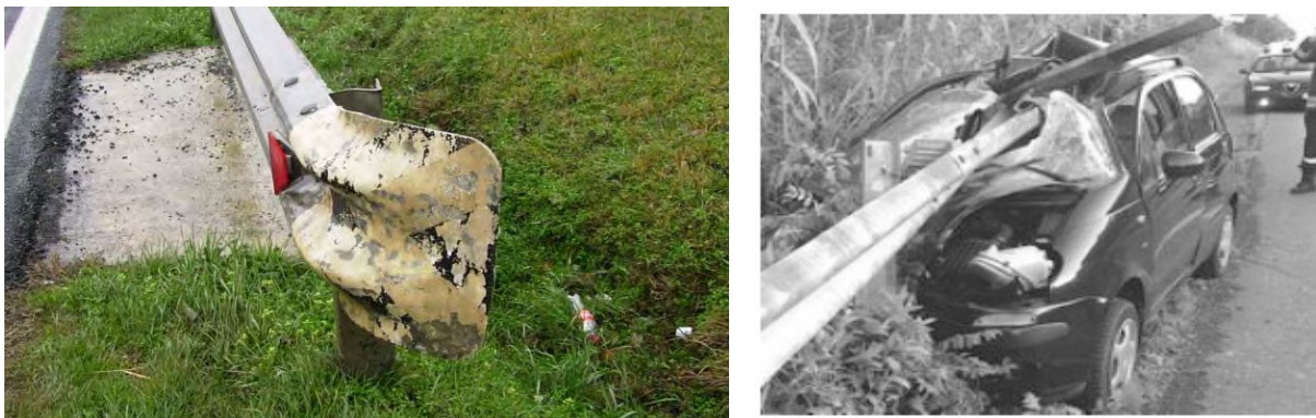
FIGURE 1 Unprotected barrier terminals (la Torre, 2011).
