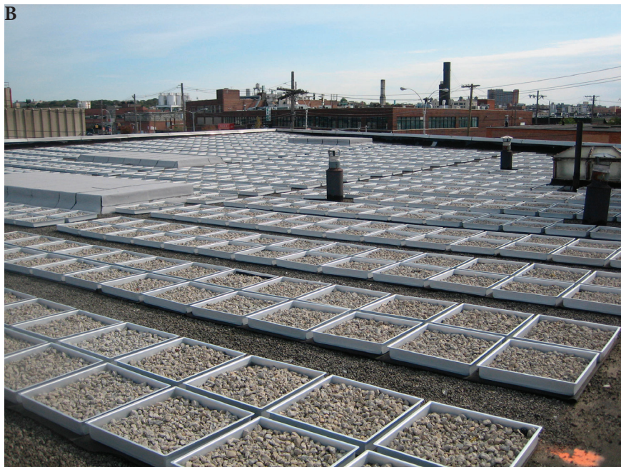
FIGURE 4 Examples of Green Infrastructure: (A) Green Roof, (B) Blue Roof, (C) Porous Pavement, (D) Bioswale
