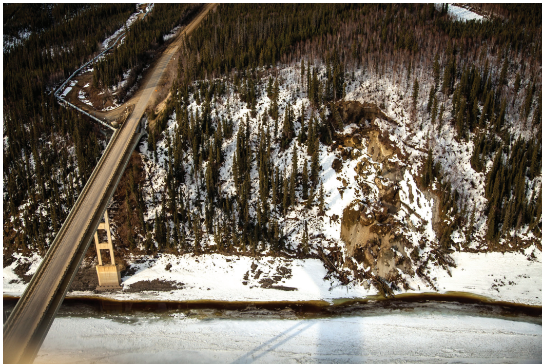
FIGURE 3.4 Permafrost slump at Yukon River Bridge, adjacent to the Dalton Highway and Trans-Alaska Pipeline System. These slumps have become more common as permafrost thaws and the surface gives way in a landslide. SOURCE: Erik Bachmann, Alaska State Division of Geological and Geophysical Surveys.
