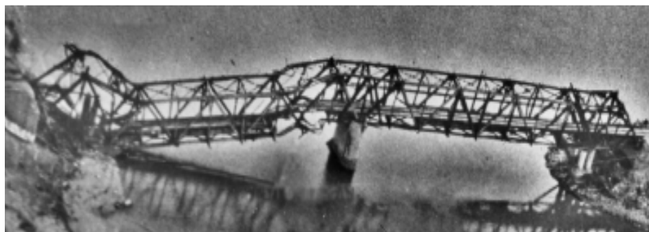
FIGURE 1-6 The Thanh Hoa (Dragon’s Jaw) bridge in Vietnam off its abutment after attack. SOURCE: See http://en.wikipedia.org/wiki/File:ThanhHoaBridge1.jpg .
