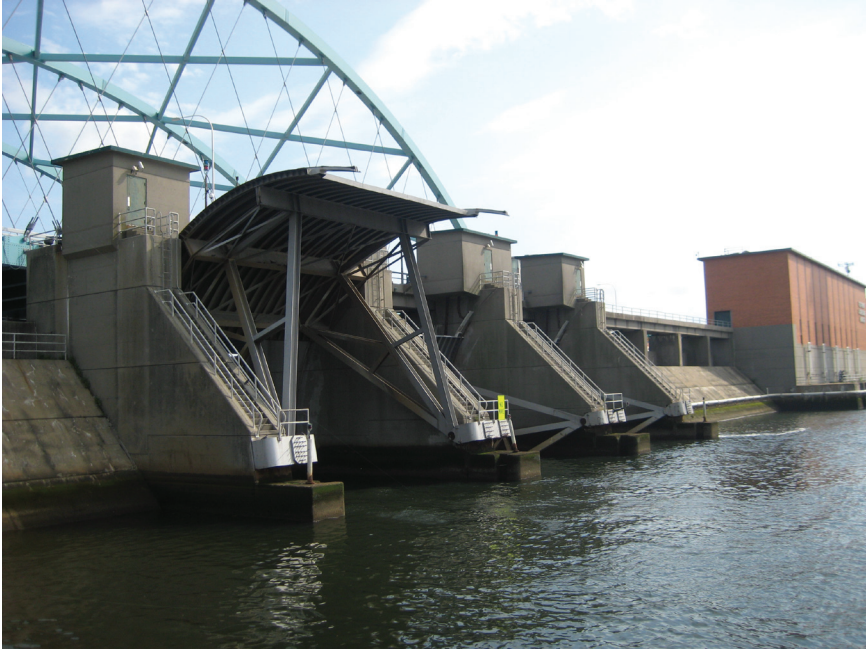
FIGURE 1-8 Fox Point hurricane barrier on the Providence River in Providence, Rhode Island, built in 1966.
