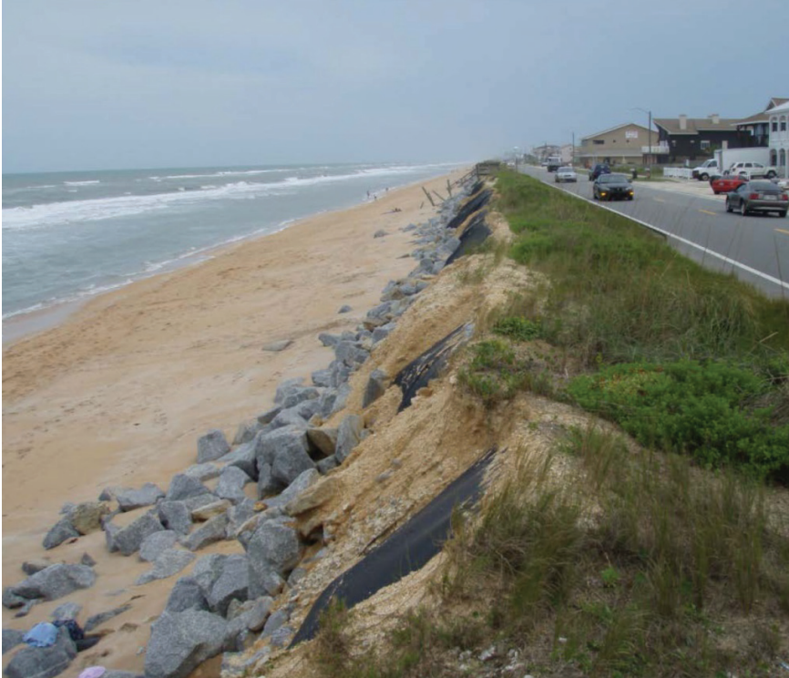
FIGURE 3-1 An eroding beach adjacent to State Road A1A in Flagler County, Florida, recently under study by the USACE for additional hurricane and storm damage risk reduction.
