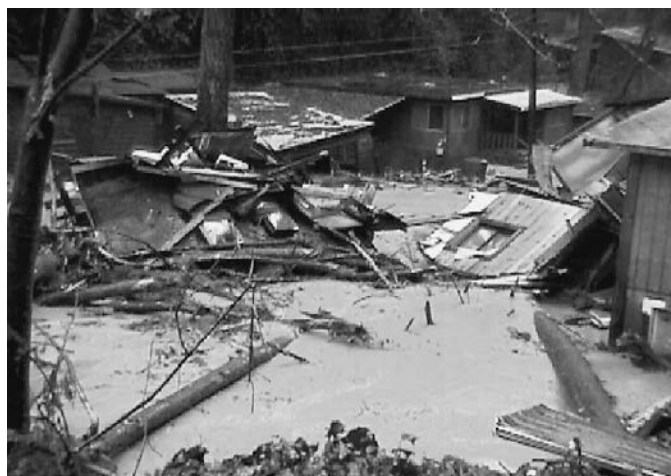
Figure 7.5. Debris generated from a flooding event in California. (Source: FEMA)
