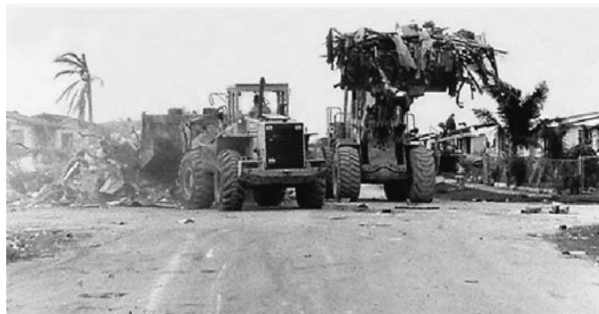
Figure 7.1. Crew using large front loaders to push debris to the curbside on a road leading to a critical facility. (Source: FEMA)
