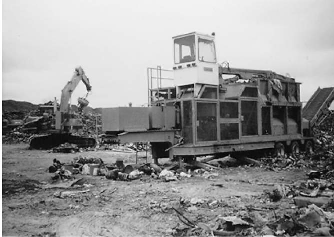
Figure 11.5. Metal maulers can be used in the metals recycling process. (Source: FEMA)
