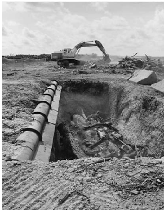
Figure 11.7. Open-air incineration pit. Note nozzles on left side. (Source: FEMA)
