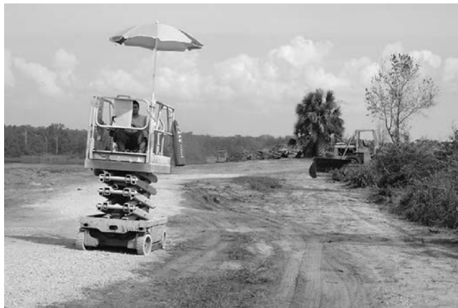
Figure 10.4. Unsafe scissor lift inspection tower. (Source: FEMA)
