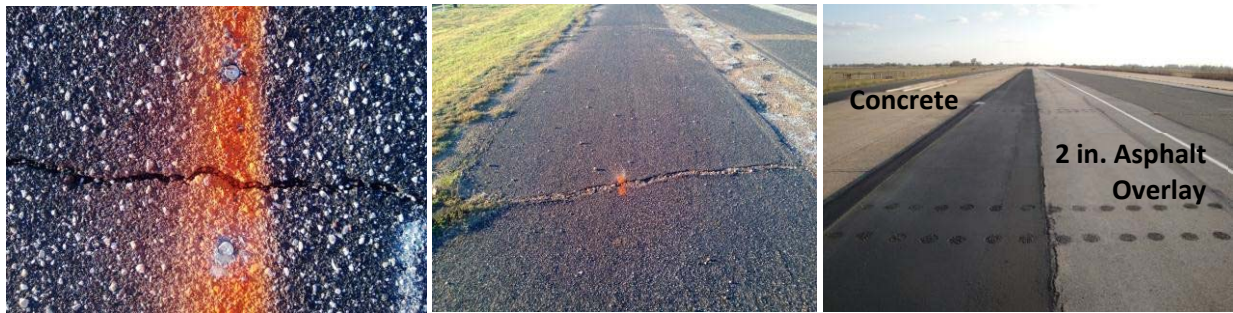
FIGURE 2 Measurement of crack movement at the Texas A&M Riverside campus (16).
