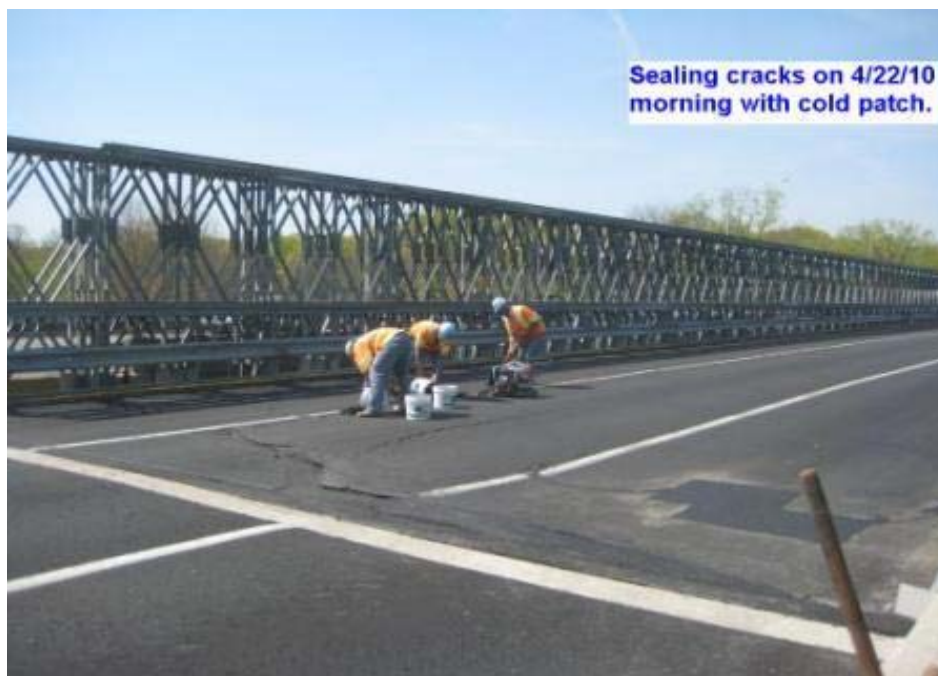
FIGURE 6 Patching of rapid deterioration on Rt. 80 ACROW bridge in New Jersey.
