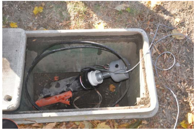
Figure 4.6. Acoustic signal injector on 4-in.-diameter pipe.
