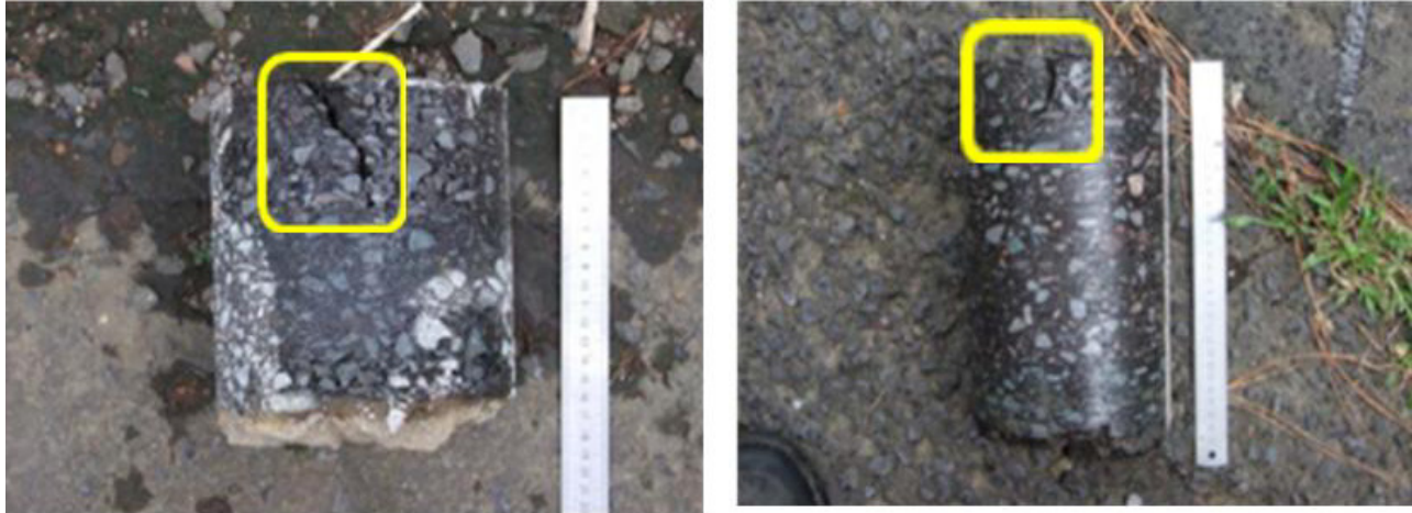
Figure 2.27. Top-down cracking in cores from Panama. Core thicknesses ranged from 6 to 12 in.
