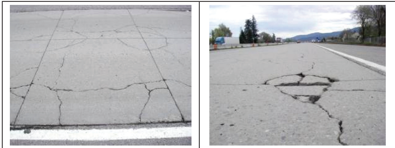
Figure 3.5. Condition of 3-in. bonded PCC overlay of HMA in 2011, following 8 years of service. Photos: WSDOT.
