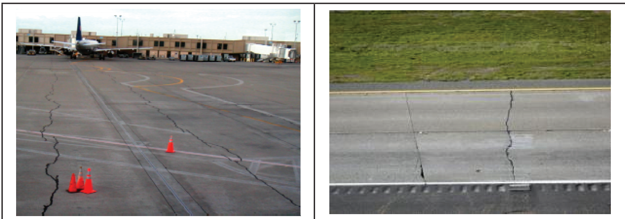
Figure 3.26. Transverse cracking on an airport apron and an Interstate highway. Photos: Joe Mahoney.
