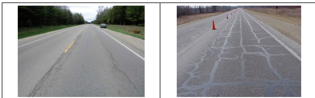
Figure 2.30. Longitudinal top-down cracking in Michigan. The photo on the right is HMA placed over rubblized PCC pavement.
