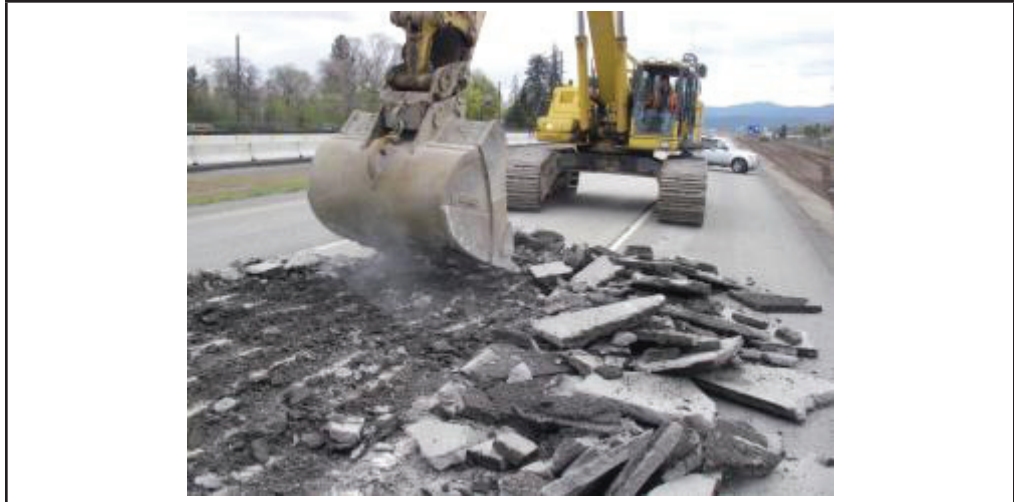
Figure 3.6. Removal of 3-in. PCC overlay before reconstruction of this portion of I-90. Bond between the PCC overlays was assessed visually during removal in 2011. Photo: WSDOT.
