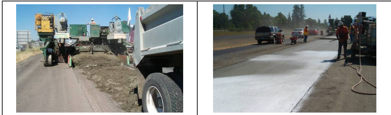
Figure 3.4. Construction of bonded PCC overlays that were placed directly on rotomilled HMA (Washington State, July 2003). Photos: WSDOT.
