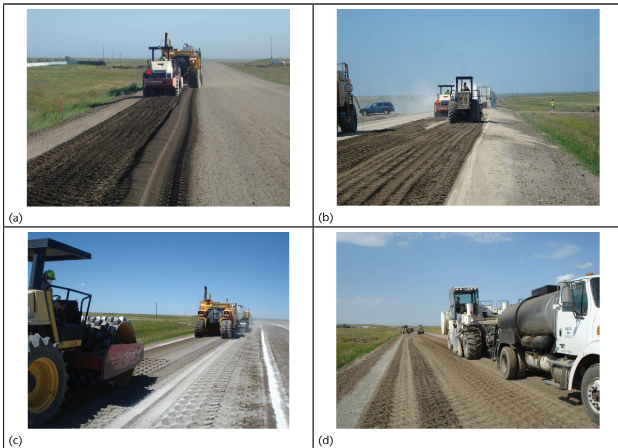
Figure 2.3. FDR construction with different stabilizing agents. (a) FDR with asphalt emulsion. (b) FDR with cement/fly ash stabilizer. (c) FDR with asphalt emulsion and dry lime. (d) FDR with foamed asphalt. Source: Bang et al., 2010.
