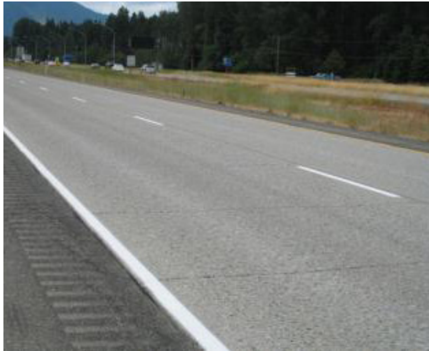
Figure 3.22. Unbonded 9-in. JPCP concrete overlay placed over concrete (I-90 in Washington State; overlay is 35 years old). Photo: WSDOT.
