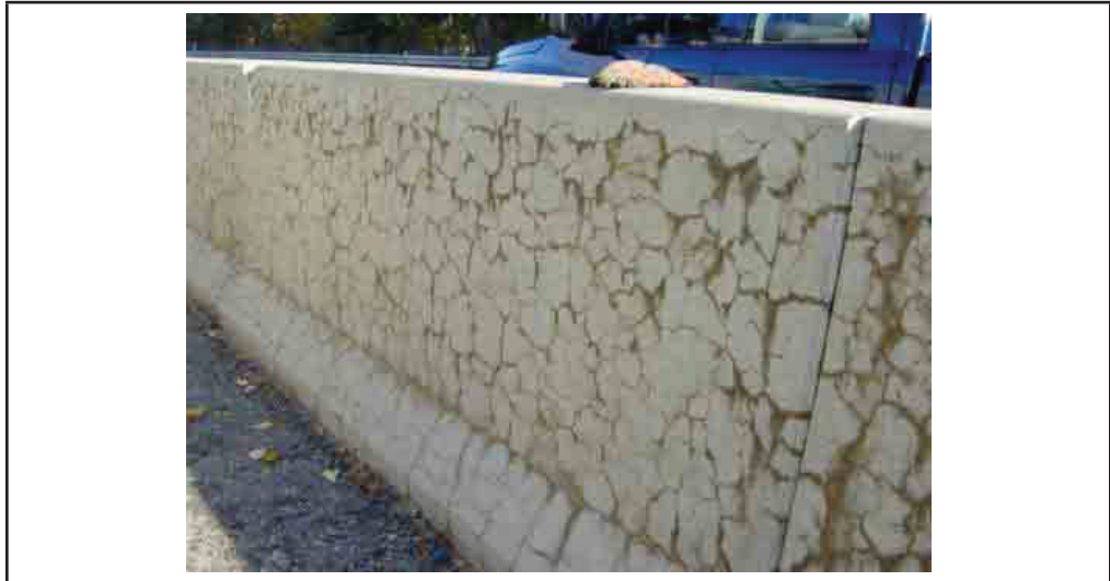
Figure 3.17. Illustration of ASR on a traffic barrier. Photo: FHWA.
