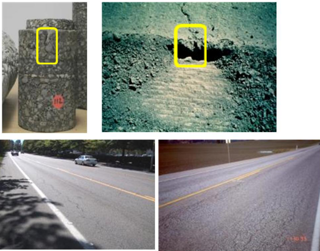
Figure 2.28. Top-down cracking in Washington State. The top photos are from Interstate 90; the bottom photos are local streets in western Washington.
