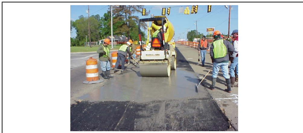
Figure 6.6. Construction of RMP. Application of the grout to the open-graded HMA. Source: Battey and Whittington, 2007.
