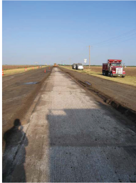
Figure 2.5. Existing concrete pavement exposed after removal of HMA layer. Source: Sebesta and Scullion, 2007.
