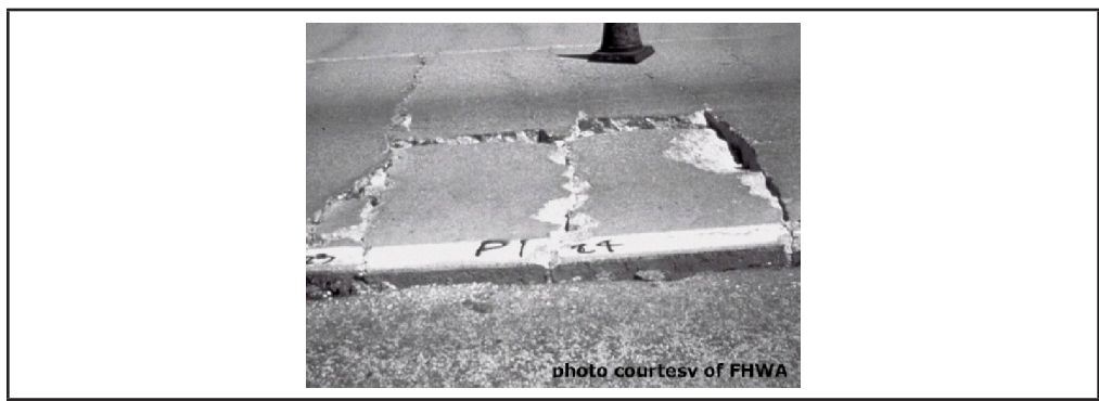
Figure 1.9. Advanced stage for a CRCP punchout. Source: FHWA.
