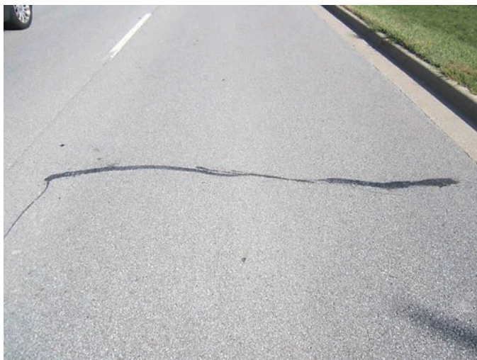
Figure 1.86. Low-severity transverse crack in Munster, Indiana.
