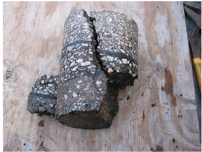
Figure 1.33. Core taken on a transverse crack to demonstrate it was reflecting from underlying pavement layers.
