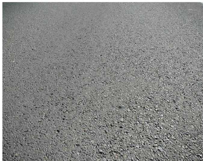
Figure 1.48. HMA surface texture in Walla Walla, Washington, at 13-month inspection.
