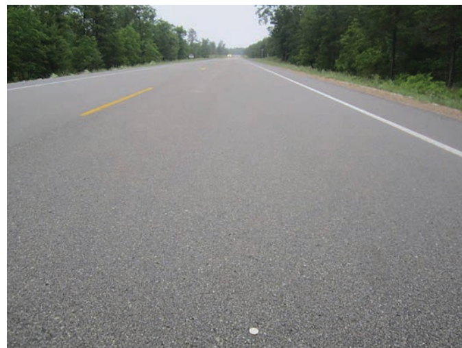
Figure 1.68. Evotherm 3G section from Rapid River, Michigan, at 22-month inspection.
