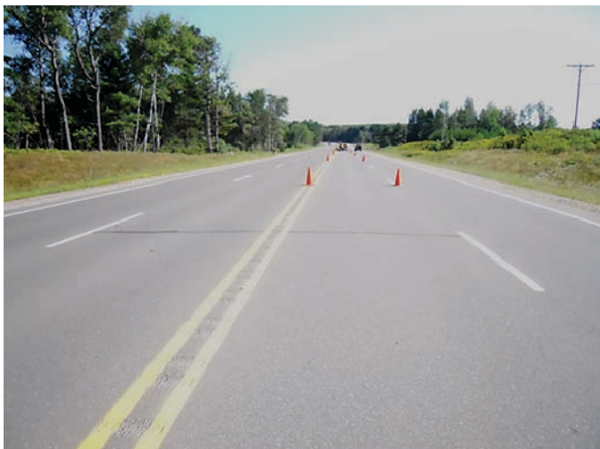
Figure 1.20. Transverse cracking in WMA section in Iron Mountain, Michigan.
