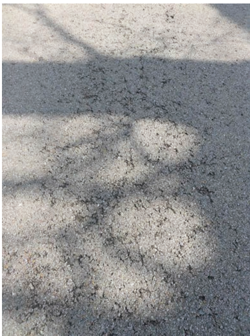
Figure 1.27. Fatigue cracking in Evotherm section in Franklin, Tennessee.
