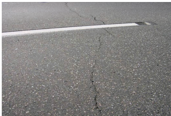
Figure 1.23. Transverse cracking in WMA section in Silverthorne, Colorado (24).
