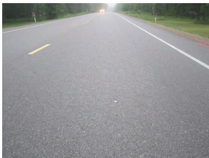
Figure 1.67. Advera section from Rapid River, Michigan, at 22-month inspection.
