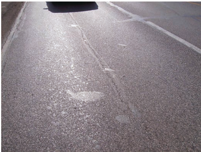
Figure 1.16. Non-wheelpath longitudinal cracking in St. Louis, Missouri.
