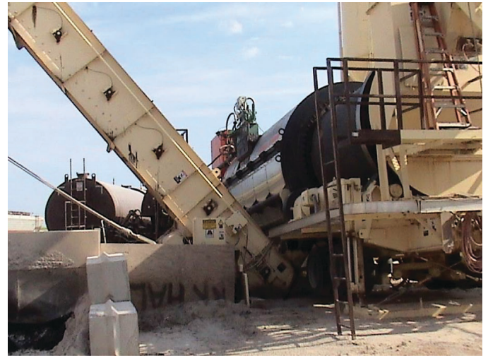
Figure 1.30. Drum and point of water injection in Graham, Texas, plant.
