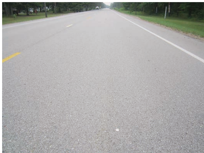
Figure 1.66. HMA control section from Rapid River, Michigan, at 22-month inspection.
