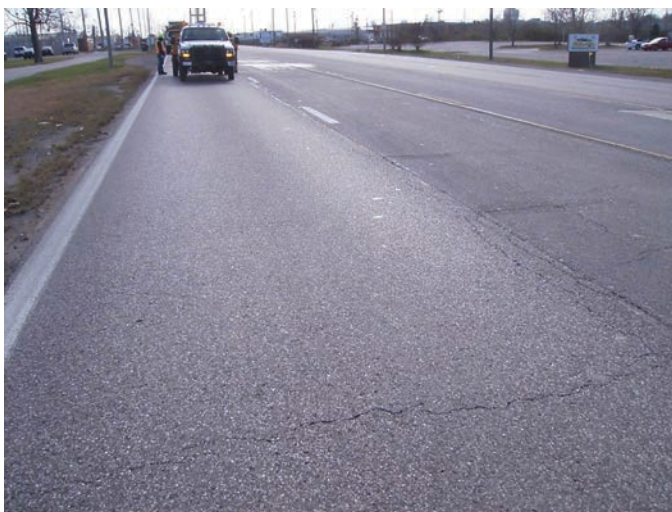
Figure 1.17. Transverse cracking in St. Louis, Missouri.
