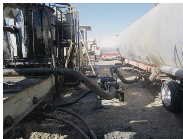
Figure 1.107. Tanks used to blend (left) and store (right) Sasobit in Casa Grande, Arizona.
