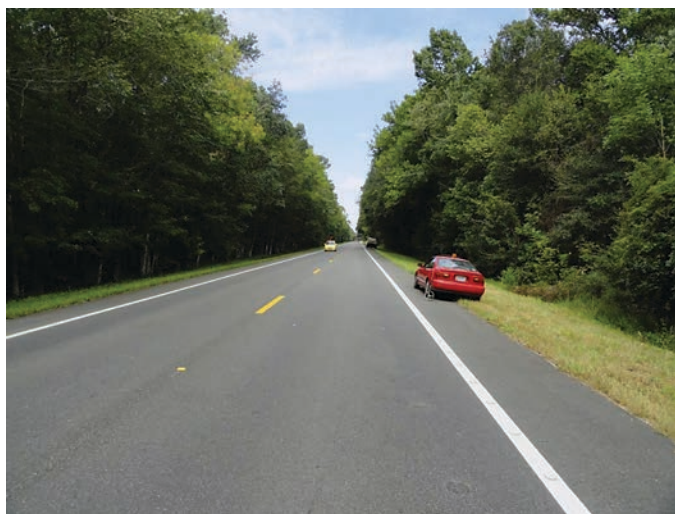
Figure 1.97. WMA (left lane) and HMA control sections (right lane) in Jefferson County, Florida.
