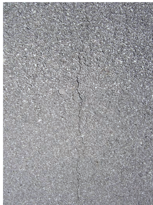
Figure 1.87. Low-severity non-wheelpath longitudinal crack in Munster, Indiana.
