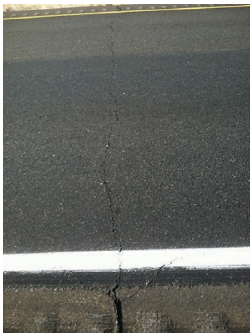
Figure 1.38. Transverse cracking in George, Washington.
