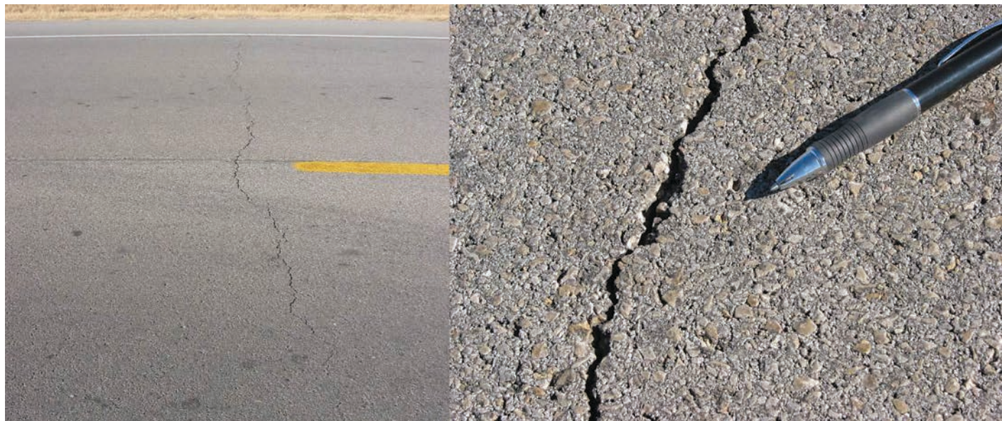
Figure 1.34. Transverse cracks on the Graham, Texas, project after 30 months.
