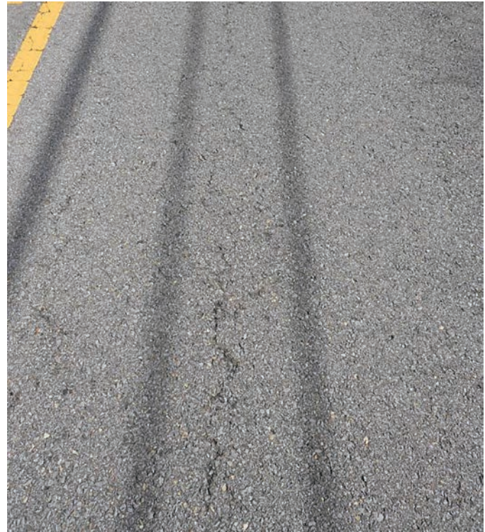
Figure 1.26. Wheelpath longitudinal cracking in Franklin, Tennessee.
