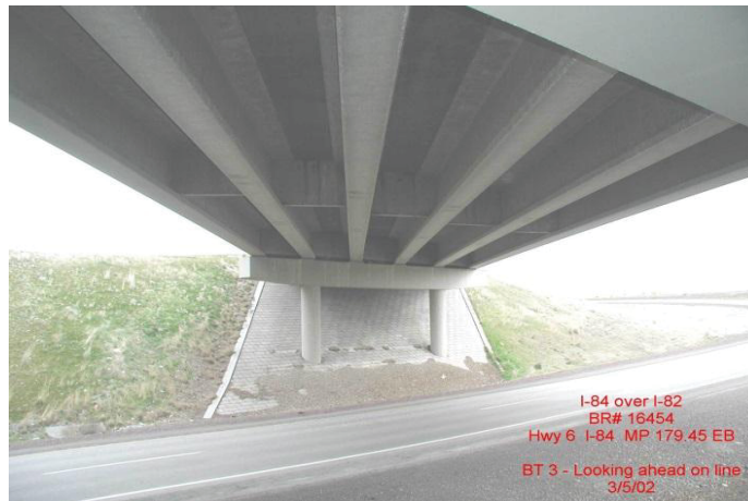
Figure 20. Condition rating history and RBI inspection interval for Bridge 16454.
