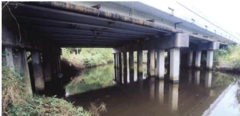
Figure 24. Example bridge in Texas with decreasing inspection interval resulting from section loss.
