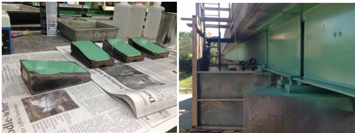
Figure B.10. Control bridge coating samples in the lab (left) and in situ testing on Exit 174, I-95, in Maine (right).
