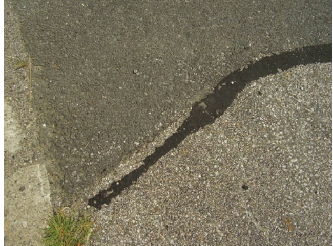
FIGURE 10 Edge seal misapplied on throw-and-roll patch (Source: R. McDaniel).
