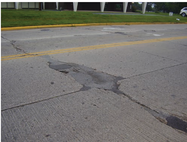
FIGURE 3 Patched concrete joint spalls (Source: R. McDaniel).
