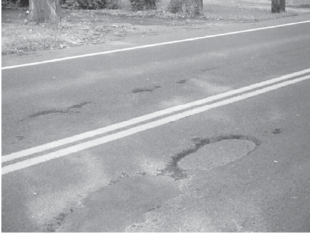
FIGURE 2 Delamination of surface layer (Source: CLRP).
