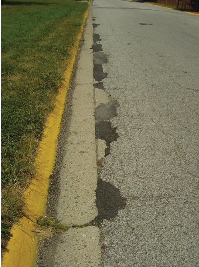
FIGURE 6 Multiple patches on asphalt pavement (Source: R. McDaniel).
