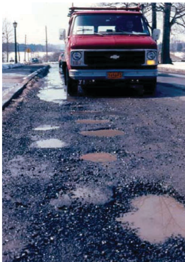
FIGURE 1 Potholes caused by poor drainage (Source: Cornell Local Roads Program, CLRP).
