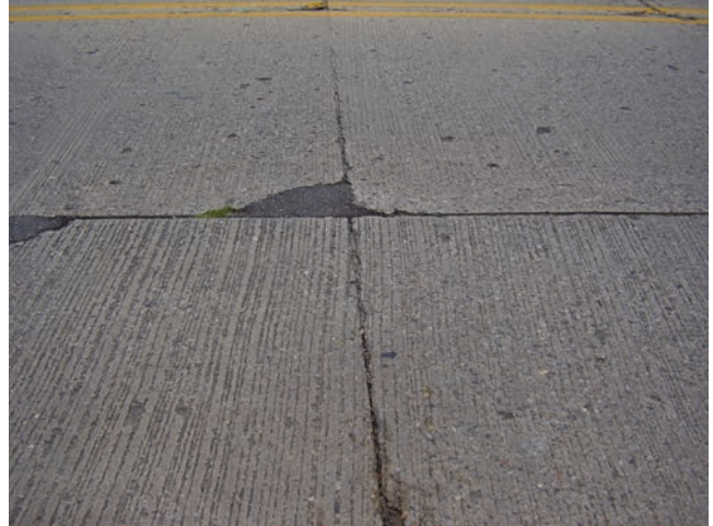
FIGURE 4 Patched corner break in concrete pavement (Source: R. McDaniel).
