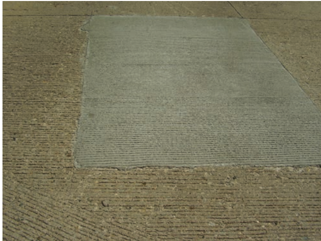
FIGURE 12 A sawed patch on concrete pavement with reinstated tining (Source: R. McDaniel).
