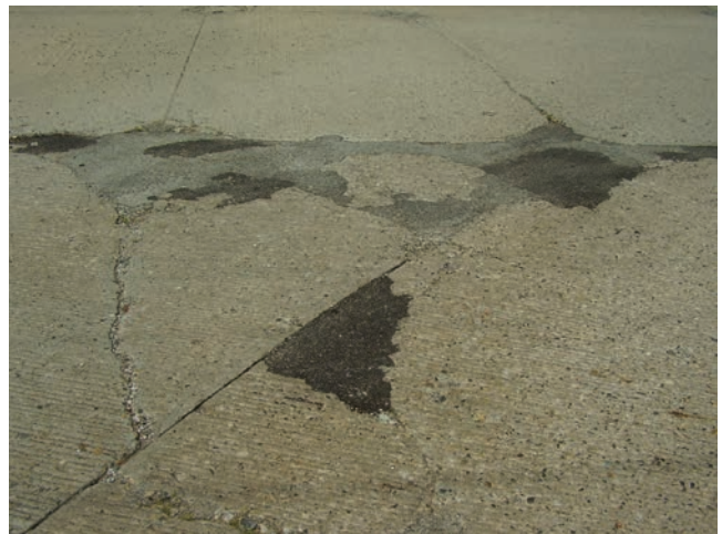
FIGURE 5 Multiple asphalt patches on concrete pavement (Source: R. McDaniel).
