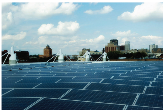
FIGURE 6 Some transit agency facilities are prime candidates to collect solar power from panels placed above maintenance yards or transit centers, such as these at Akron Metro purchased with federal capital grants ( Source : Akron Metro website).
