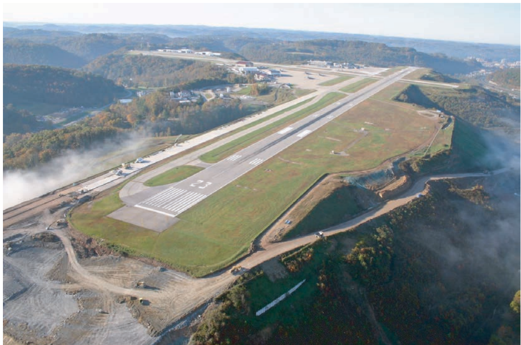
FIGURE 17 Aerial view of Yeager Airport during the extension of Runway 23 and widening of Taxiway A. (Source: Yeager Airport.)
