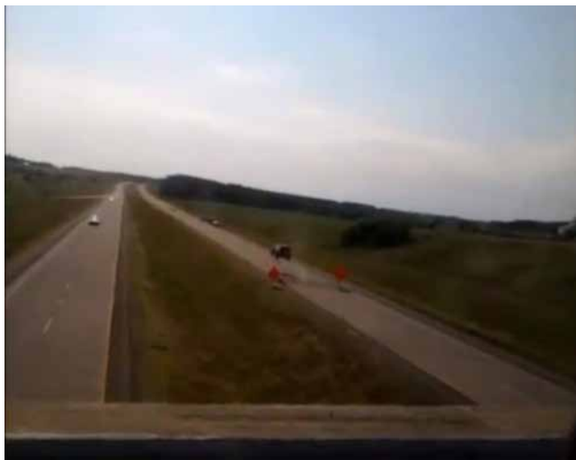
FIGURE 21 Vehicle goes airborne after hitting a heat-buckling site on State Highway 29 Chippewa Falls, Wisconsin, in 2012 (Courtesy: Theresa L. Reich).
