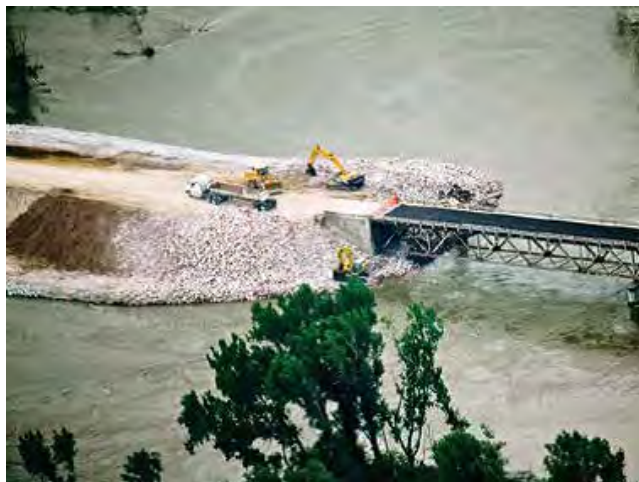
FIGURE 5 Crews at work on the IA-175 Missouri River bridge at Decatur, Nebraska, 2011 (IDOT).
