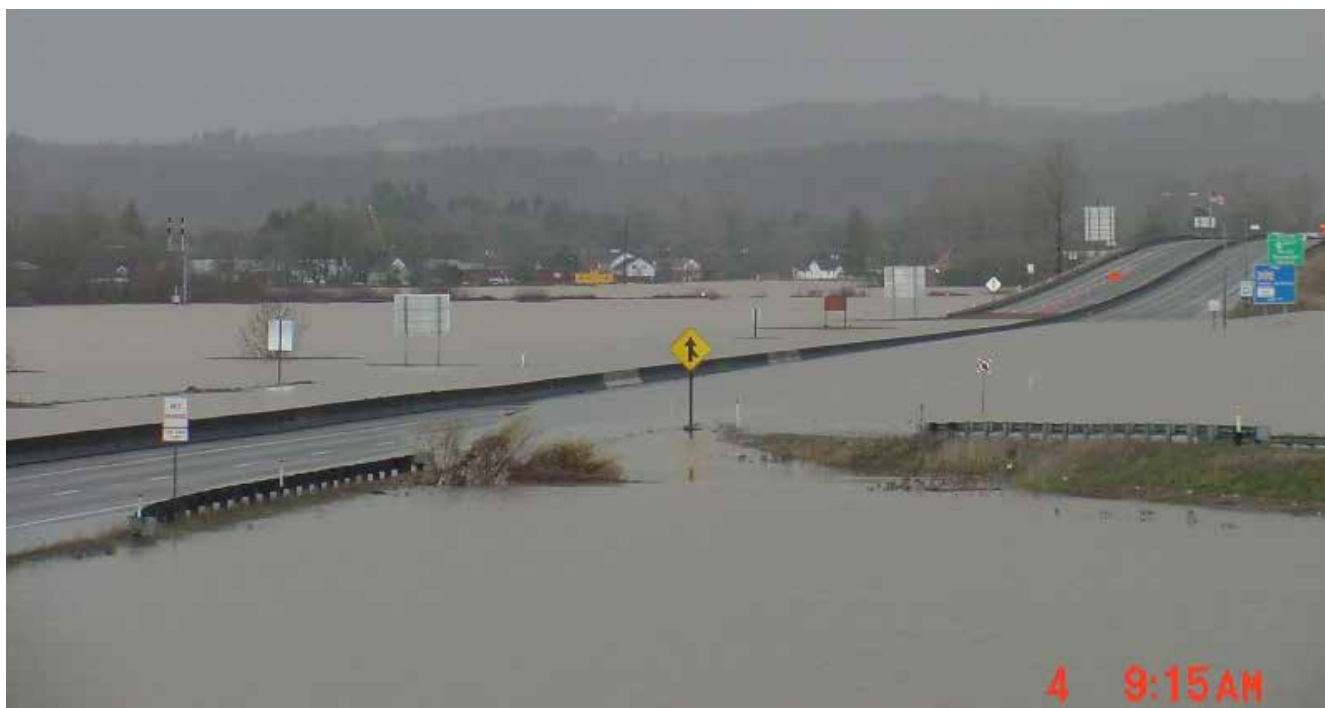
FIGURE 10 Flooding on Interstate 5 in Chehalis, Washington, December 4, 2007 (Flickr Commons, WSDOT).
