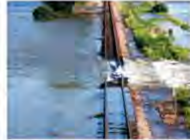
This railroad track along IA 2 near I-29 and the Council Bluffs levee is in an area that was particularly hard-hit.
