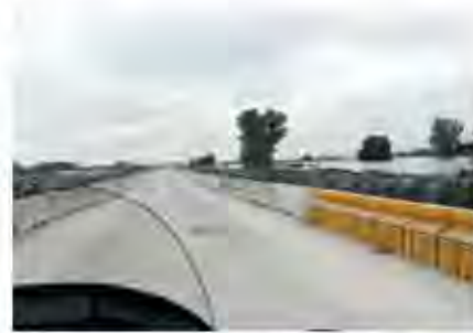
A flood barrier wall installation on a section of I-29 in Macon County.
