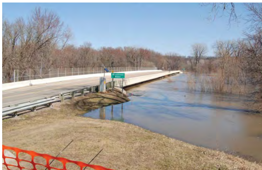
PHOTO: NCHRP Web-Only Document 175, EVALUATION OF BRIDGE SCOUR RESEARCH—PIER SCOUR PROCESSES AND PREDICTIONS
