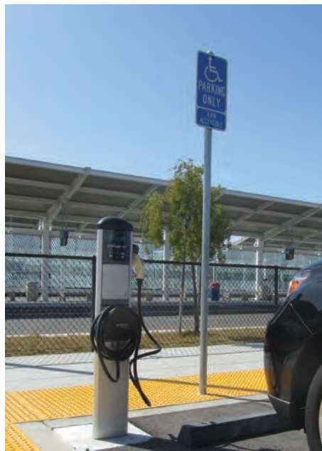
FIGURE 8 EV-charging ADA-compliant parking space at Oakland International Airport. (Source: LeighFisher September 2013.)
