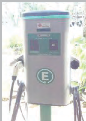
Dual-port EV charging station at Honolulu International Airport
