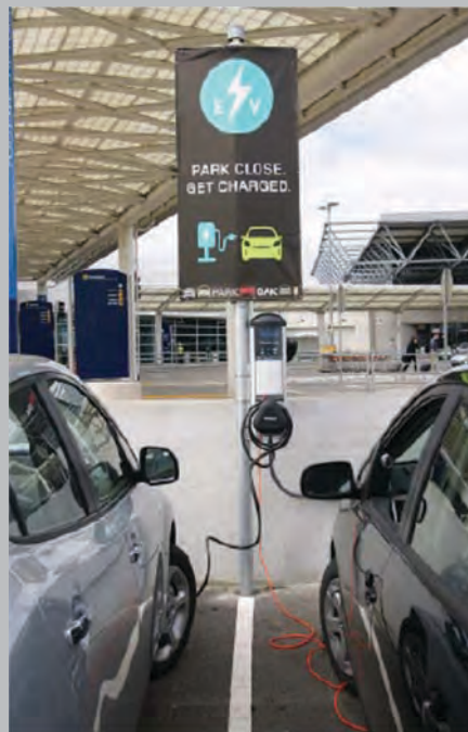
EV charging station, Oakland International Airport
