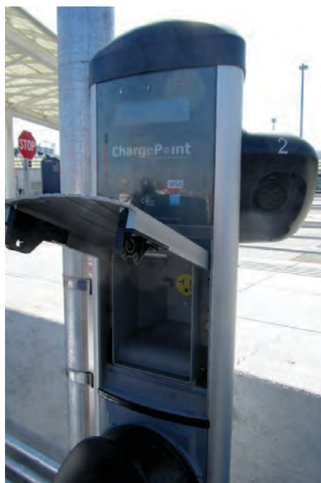
FIGURE 6 Dual-port Level 1/2 EV charging station. (Source: LeighFisher September 2013.)
