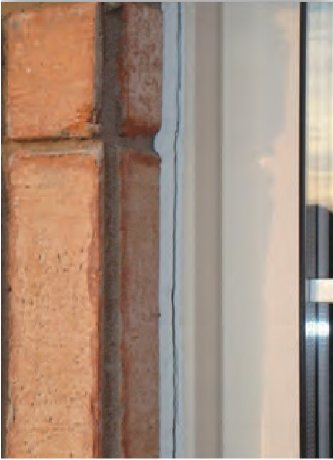
Figure 7-1. Crack in sealant.
