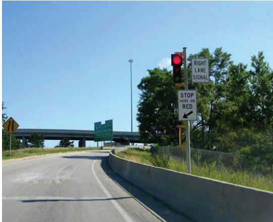
Figure 4.13. Ramp metering installation (right-lane signal).
