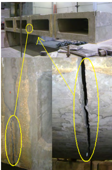
Figure C.26. Side (bottom left) and underside (bottom right) cracking.
