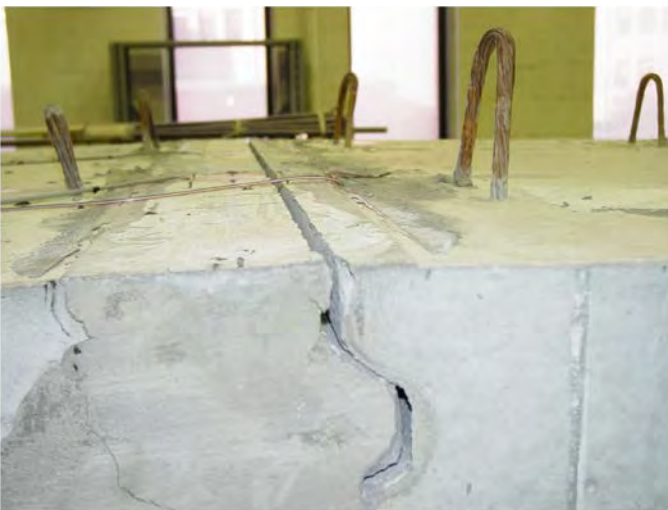
Figure 3.93. Crack at the closure region due to tensile force over the interior support.
