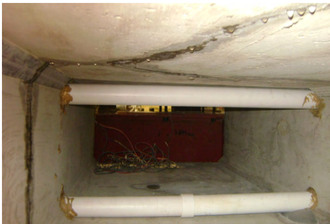
Figure C.23. Interior view of cracking at flange along northeast side of joint.
