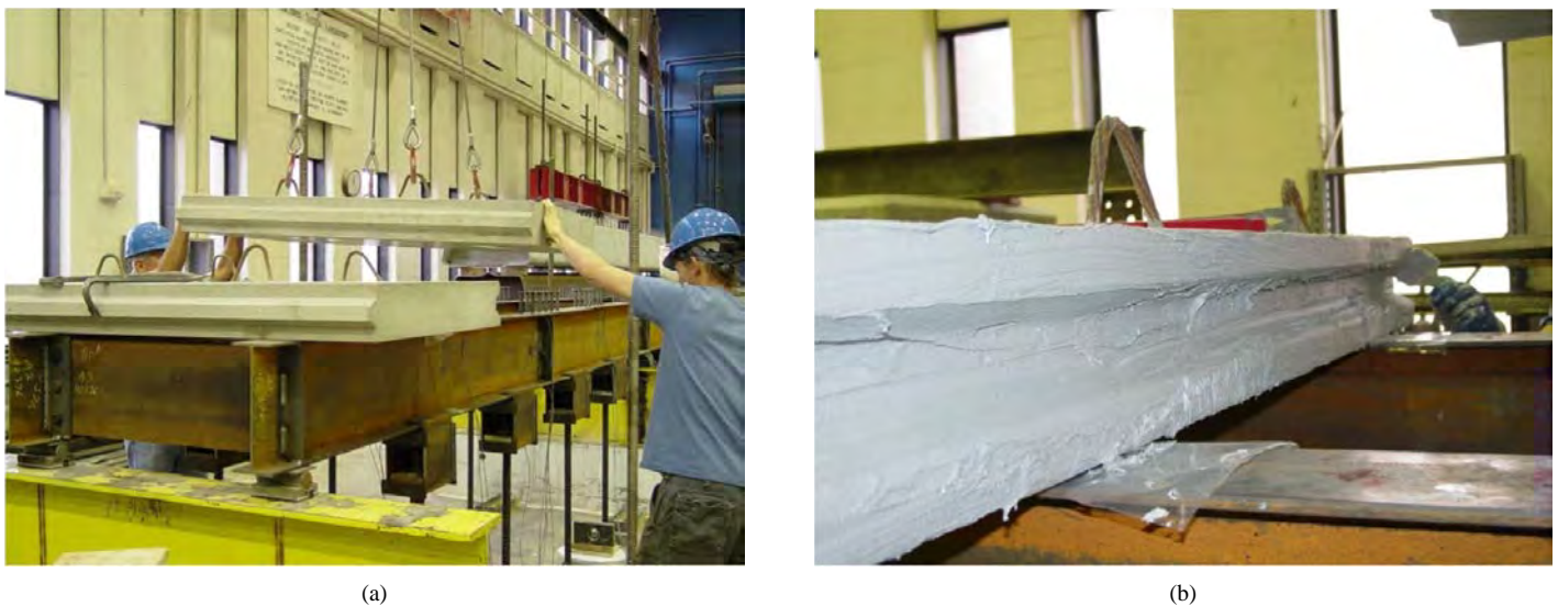
Figure 3.86. (a) Placing precast concrete panels and (b) high-strength epoxy spread over the match-cast shear key.
