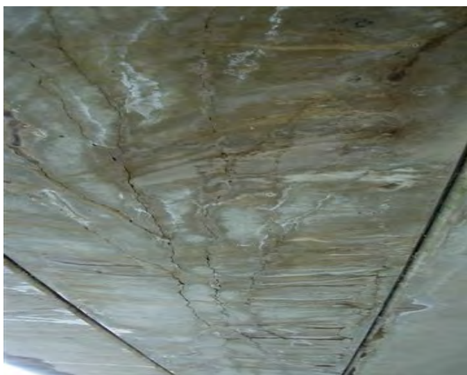
Figure C.2. Crack developed in adjacent box beam bridges.
