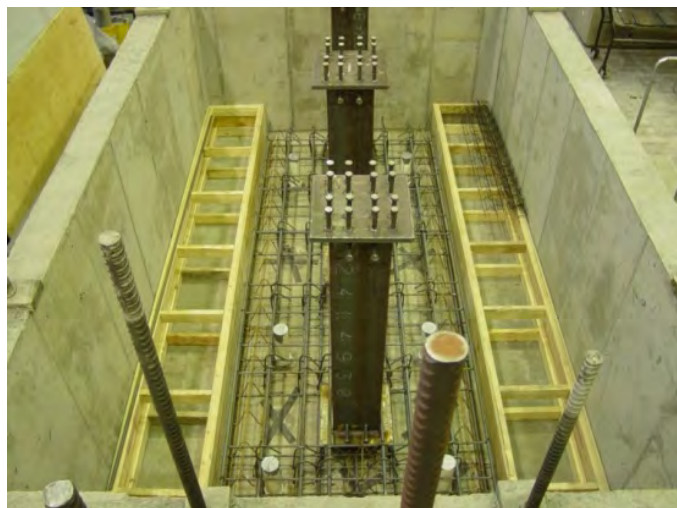
Figure 3.55. Concrete box, three small piles, concrete forms for the bottom slab, and the bottom slab reinforcement.
