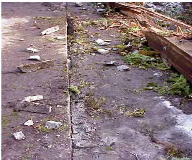
Figure C.1. Crack developed in joint between adjacent box beams.
