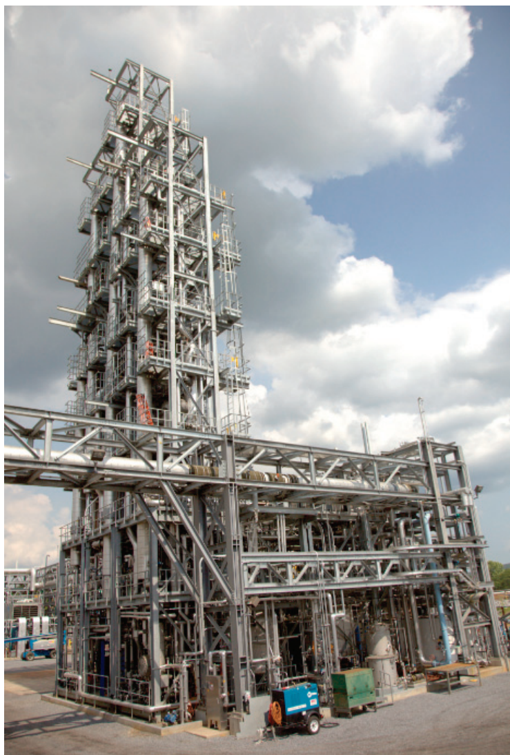
FIGURE 3.6 Conventional amine solvent plant for CO 2 separation at the National Carbon Capture Center in Wilsonville, Alabama. This is a demonstration plant that bridges technologies from the bench scale to the pilot scale, and the absorber unit that is currently in place captures 3,650 tCO 2 /yr. In contrast to the air contactor used for extremely dilute air capture, this flue-gas contactor (absorption column) can be tall for increased CO 2 separation due to the inherent driving force of the flue-gas stream. This image provides an example for dimensional comparison to the DAC plant in Figure 3.5, not a comparison of scale as the annual removal rate by the National Carbon Capture Center is small since it is for demonstration purposes only. SOURCE: Courtesy of Frank Morton, Business Development Manager of the National Carbon Capture Center, Southern Company.
