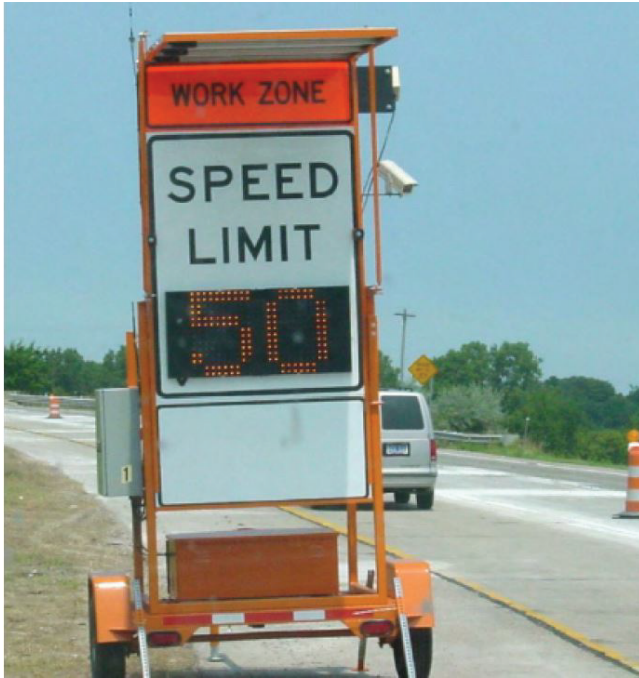
FIGURE 10 Trailer-mounted changeable speed limit (CSL) sign (MinnDOT 2008).
