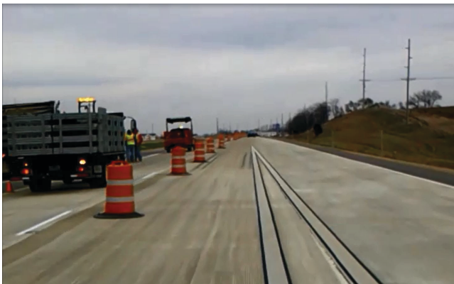
FIGURE 15 Restriction of expressway lane width, possibly initiated by a contractor attempting to reduce speeds adjacent to the activity area (Rizos 2014).
