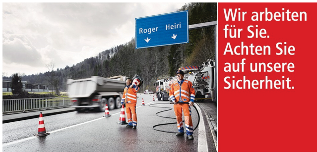
FIGURE 47 A Swiss work zone public information website puts the emphasis on protecting the safety of individual workers ( Wir arbeiten für Sie 2014). This is one of a series of images that display workers' first names on overhead sign gantries (in this case Roger and Heiri/Harry). The tag line translates, "We work for you. Look out for our safety."
