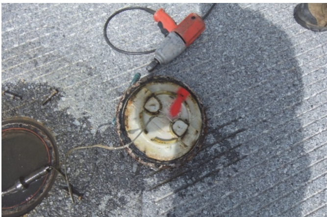
Figure 23. Primary cabling flooded by storm water.
