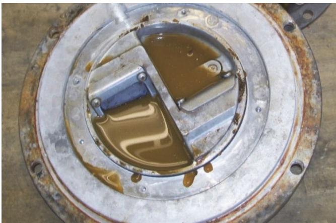
Figure 26. Water inside light fixture.
