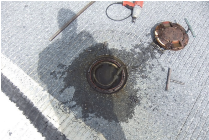
Figure 22. Water surging through lighting infrastructure.
