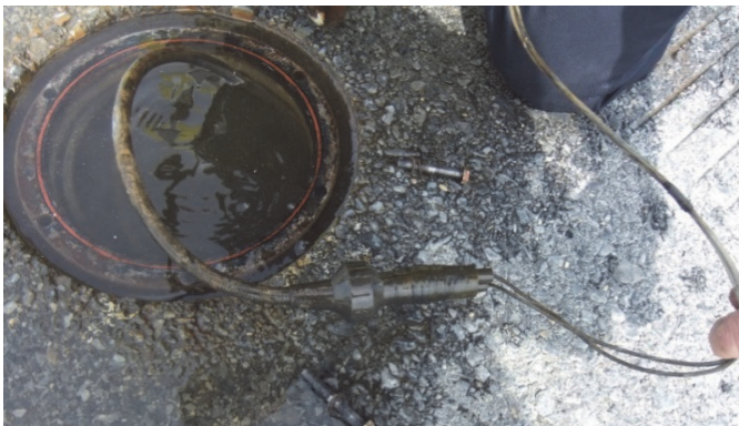
Figure 24. Accumulation of silt and corrosion on cabling.
