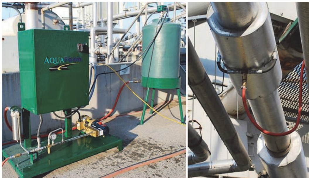
Figure A-40. Asphalt foaming system at Manatts, Inc. plant.
