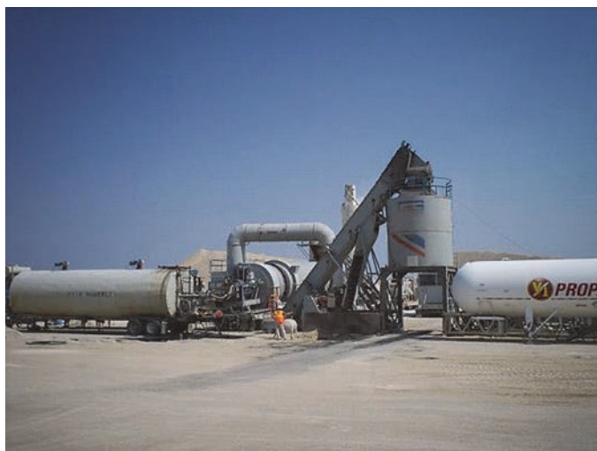
Figure A-25. Asphalt plant at the Wyoming field site.
