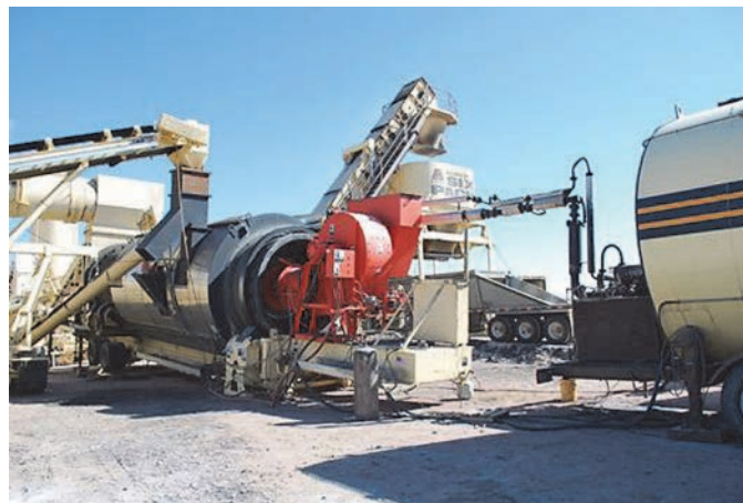
Figure A-34. Counter-flow drum at Commercial Asphalt Inc. plant in South Dakota.
