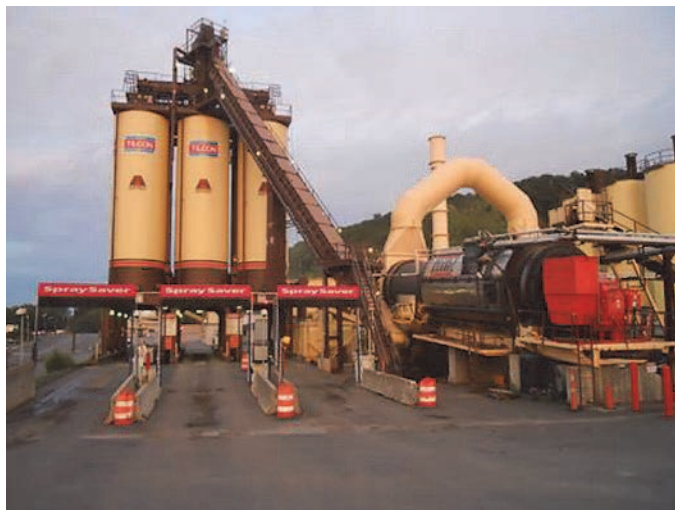
Figure A-22. Tilcon asphalt plant.
