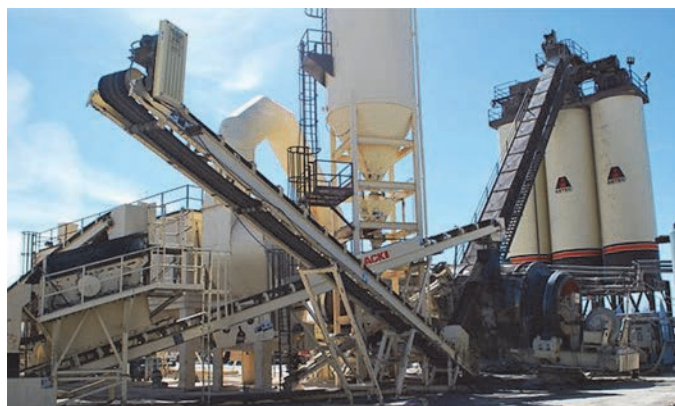
Figure A-4. RTI hot mix plant located in Buda, Texas.
