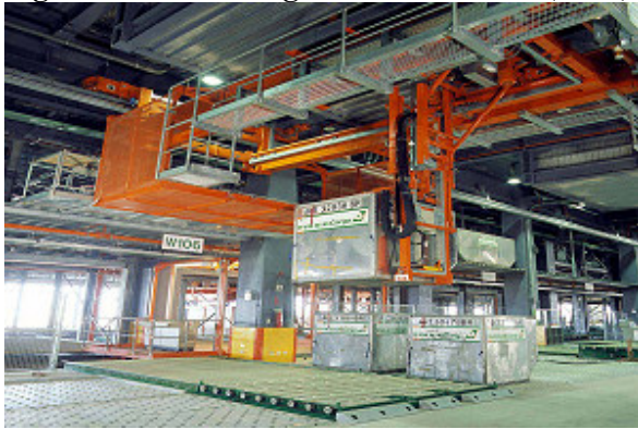
Figure 4-15 Elevating Transfer Vehicle (ETV) Systems. (SOURCE: Lynxs Group.)
