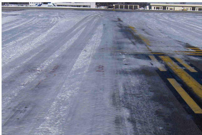
FIGURE 16 Example of obscured runway hold and taxiway centerline markings. Photo credit: S. Quilty, SMQ Airport Services.
