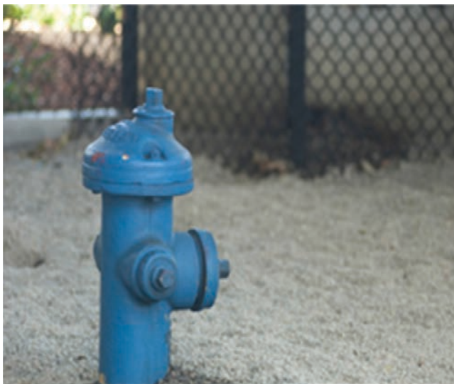
FIGURE 21 Fire hydrant in SFO SARA (SFO photo).
