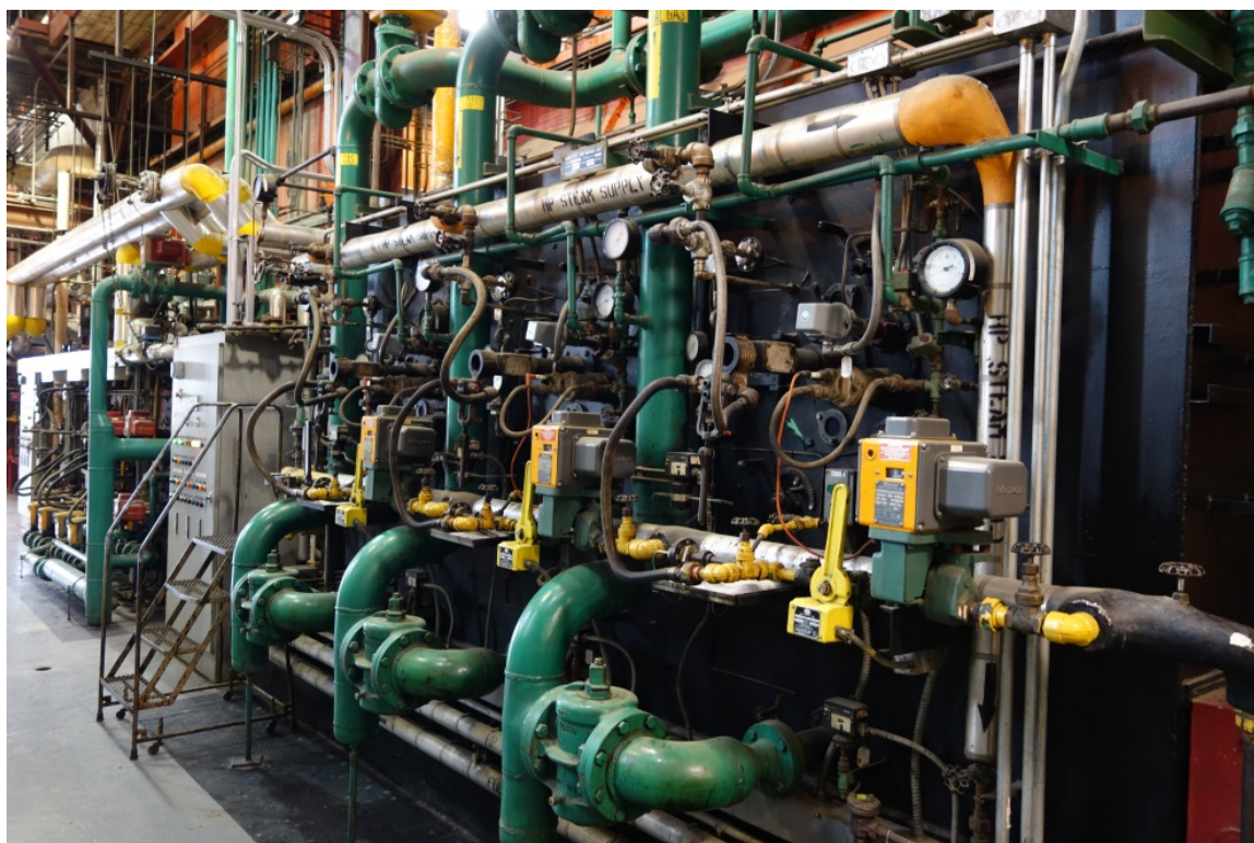
Figure 2. Boilers at Boston Logan Central Plant.
