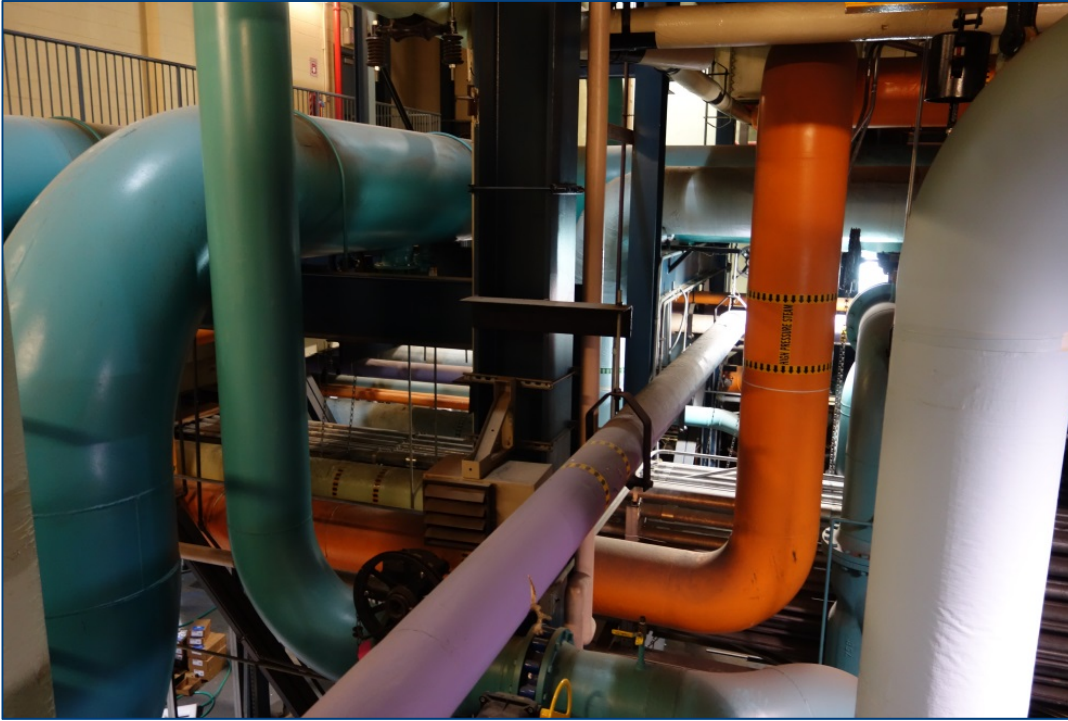
Figure 5. Distribution Systems in Boston Logan Central Plant.
