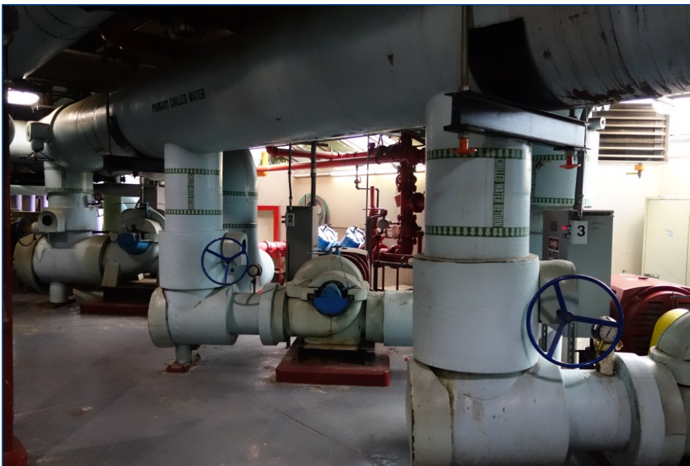
Figure 4. Chilled Water Pumps at Boston Logan Central Plant.
