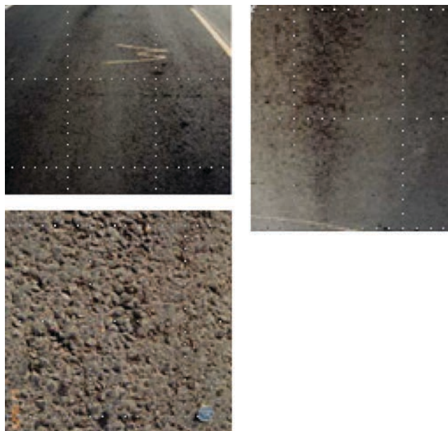
FIGURE 10 Example of moderate level of segregation [Source: Gavin and Heath (2002)].
