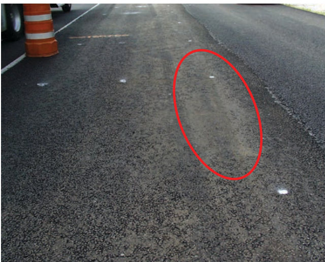
FIGURE 5 Example of random segregation (separation of binder and stone) in SMA [Source: Stroup-Gardiner (2014)].
