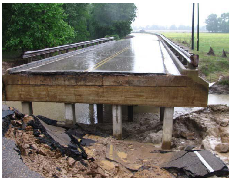
FIGURE D - 48: Example of Structural Damage during the May, 2010 Flood Event. Courtesy: TDOT.
