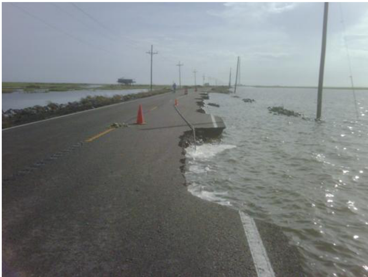
FIGURE D - 64: Hurricane Isaac, 2012 – Damage to LA 1 – South of Fourchon Road to Grand Isle, Louisiana. Courtesy: Louisiana DOTD.
