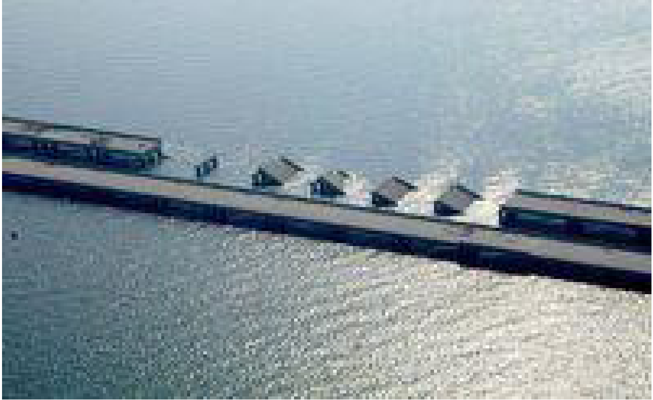
FIGURE D - 66: Hurricane Katrina, 2005 – Damage to I-10 Causeway. Courtesy: Louisiana DOTD.
