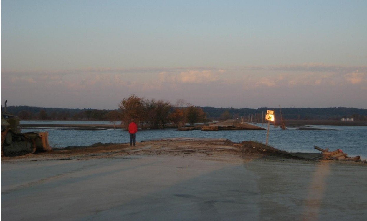
FIGURE D - 13: Scour location immediately after occurrence of scour. Courtesy: Missouri DOT.
