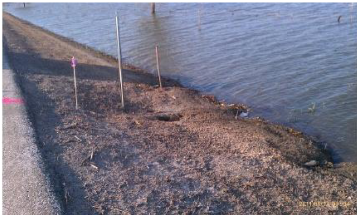
FIGURE D - 8: Culvert with Joint Separation. Courtesy: Iowa DOT.
